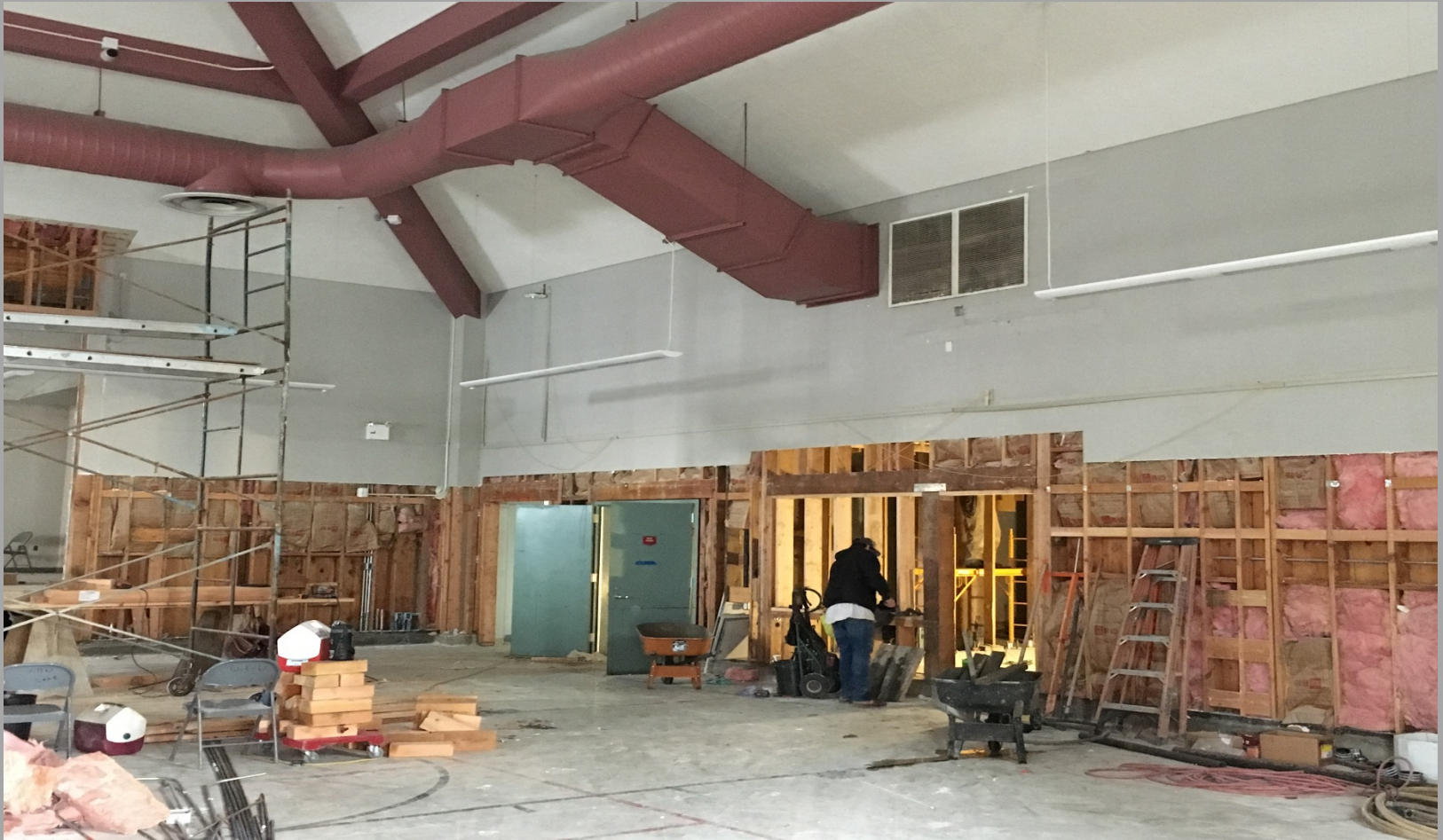
View of Demolition Completion & New Framing Inside of Building E – Looking Northeast toward Former Kitchen
