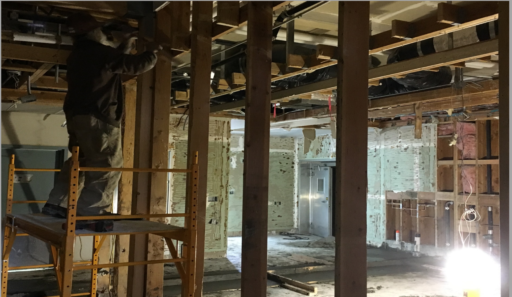
View of Demolition Completion & New Framing in Former Kitchen Inside of Building E
