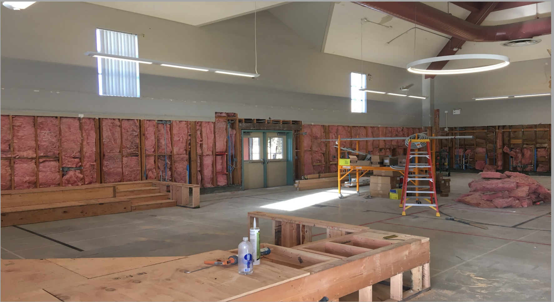
View of Modernization Work @ Building E; Reading Nook Stadium Seating in Foreground - Looking Northwest
