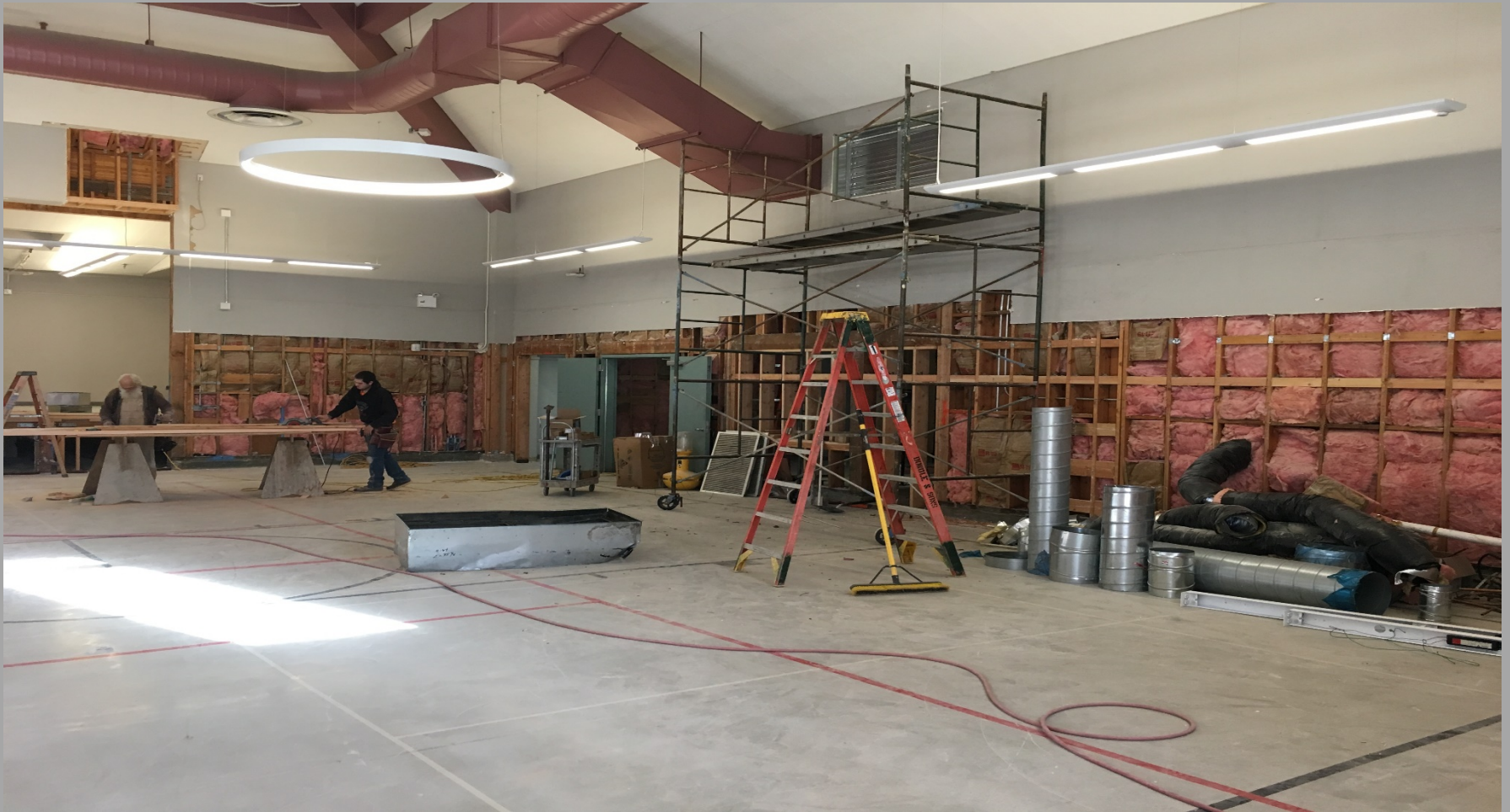
View of Modernization Work @ Building E - Looking Northeast toward New Book Storage Room & Hallway Entrance
