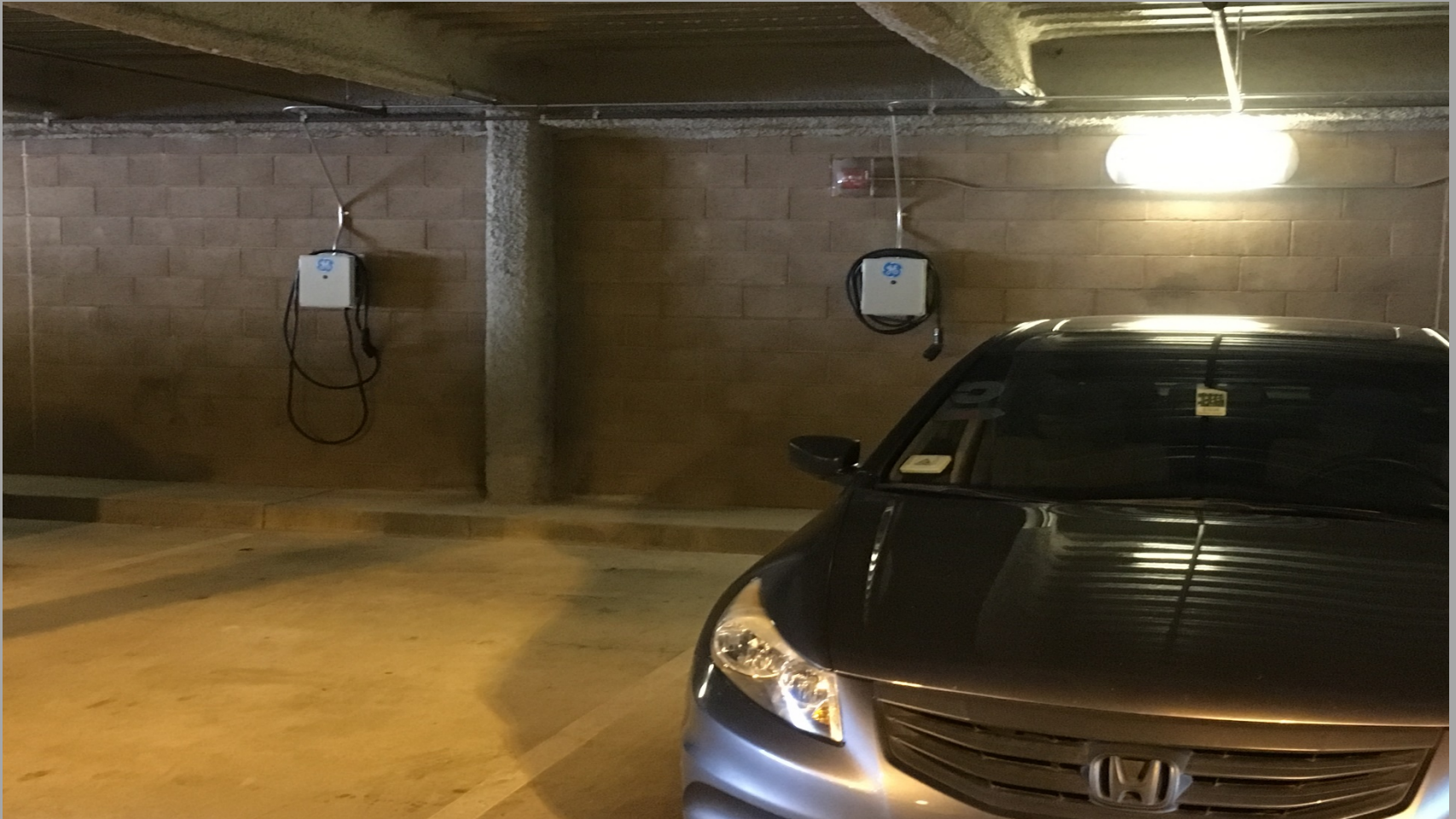
View of New EV Charging Stations in Parking Garage @ Marina Vista Elementary School
