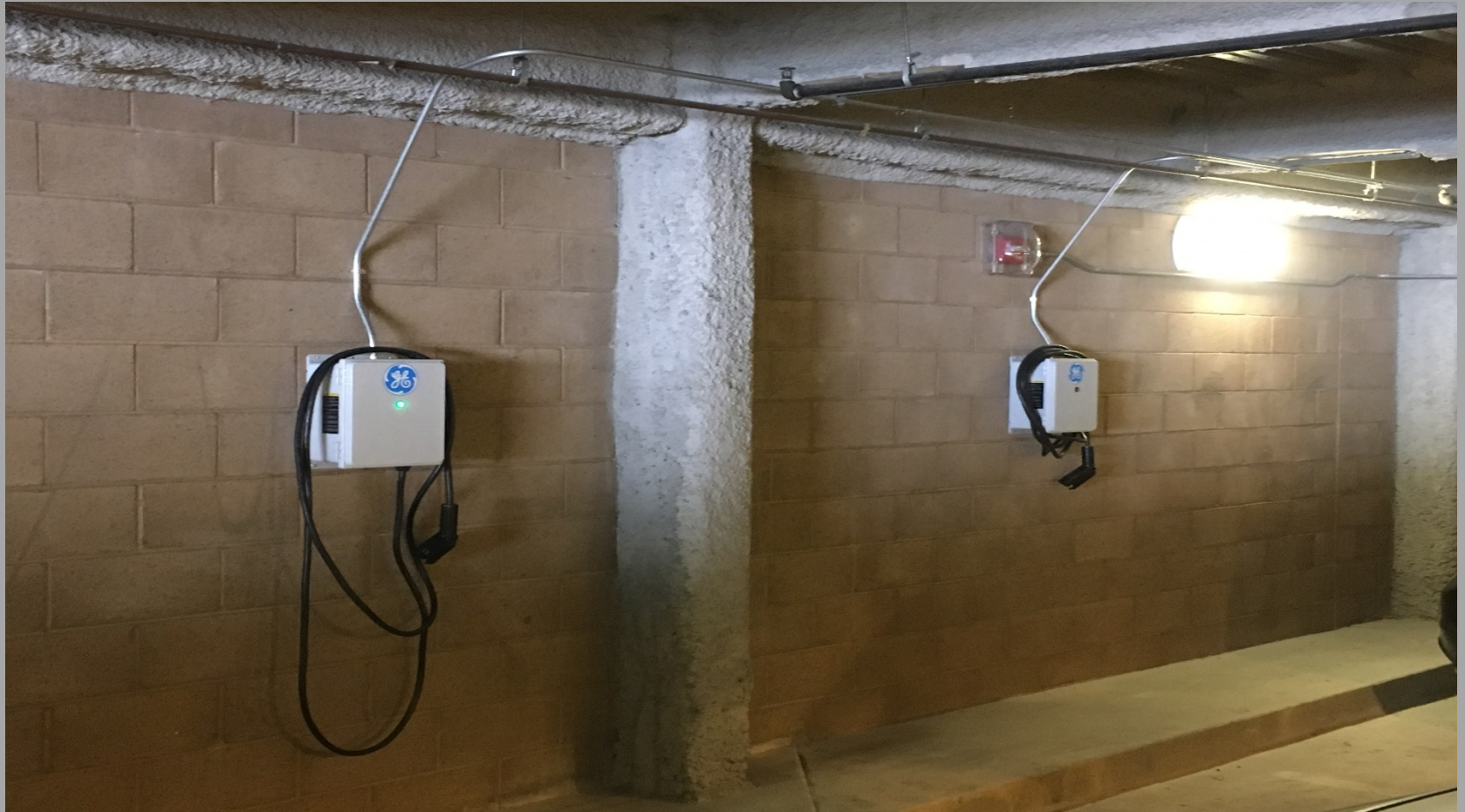
View of New EV Charging Stations in Parking Garage @ Marina Vista Elementary School
