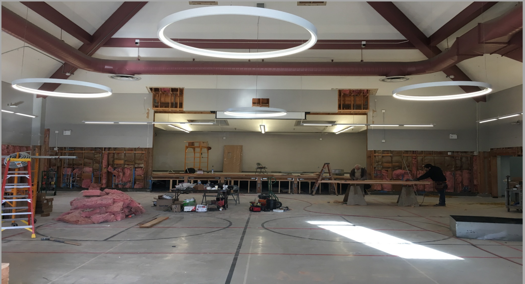
View of Modernization Work @ Building E - Looking North toward New Computer Lab. @ former Stage
