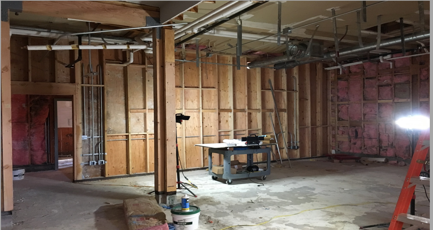
View of New Framing in former Kitchen/New Book Storage Room @ Building E - Looking Southeast
