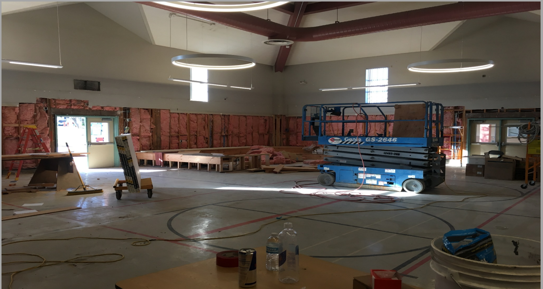
View of Modernization Work @ Building E - Looking Southwest toward Reading Nook Stadium Seating
