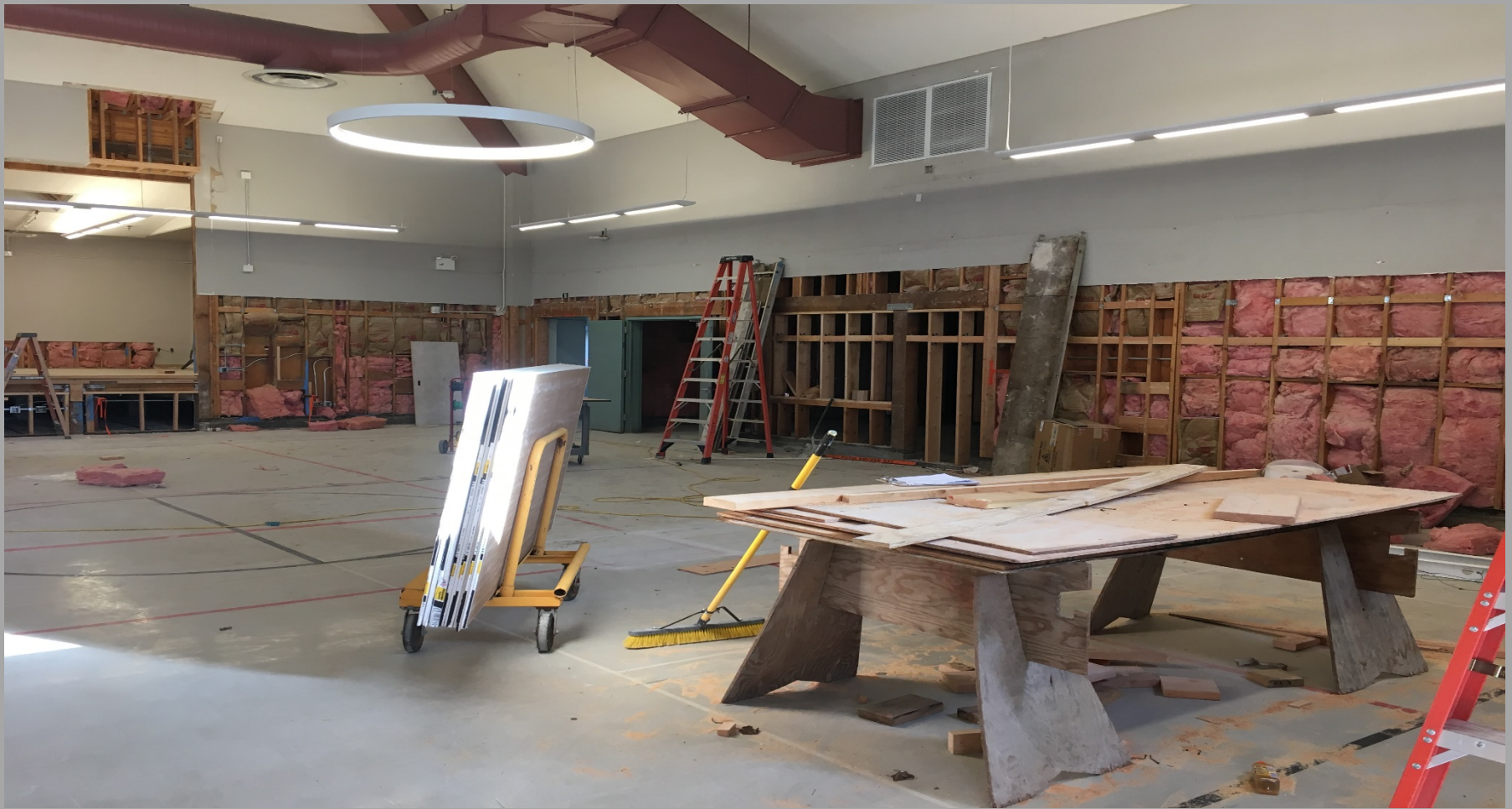
View of Modernization Work @ Building E – Looking Northeast toward Hallway & New Book Storage Room
