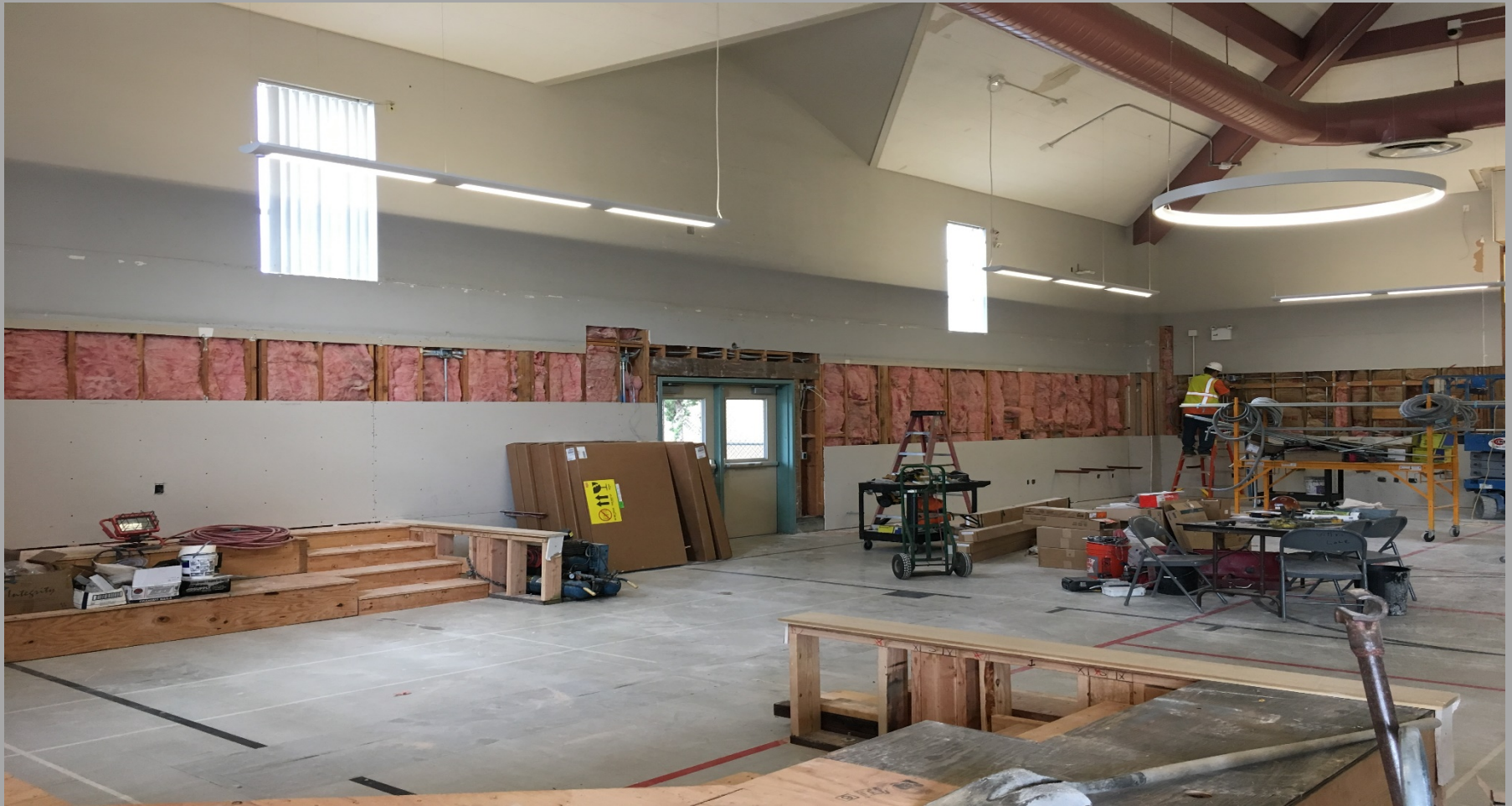
View of Modernization Work @ Building E - Looking Northwest toward Check-Out Counter Location
