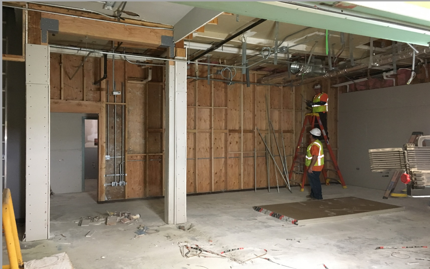
View of Electrical Work Inside of New Book Storage Room @ Building E
