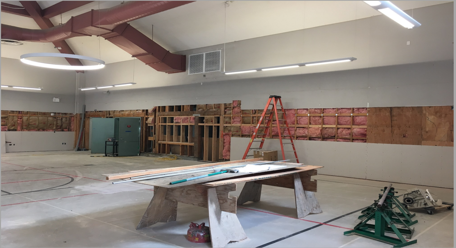
View of Modernization Work @ Building E - Looking Northeast toward Hallway & Book Storage Room
