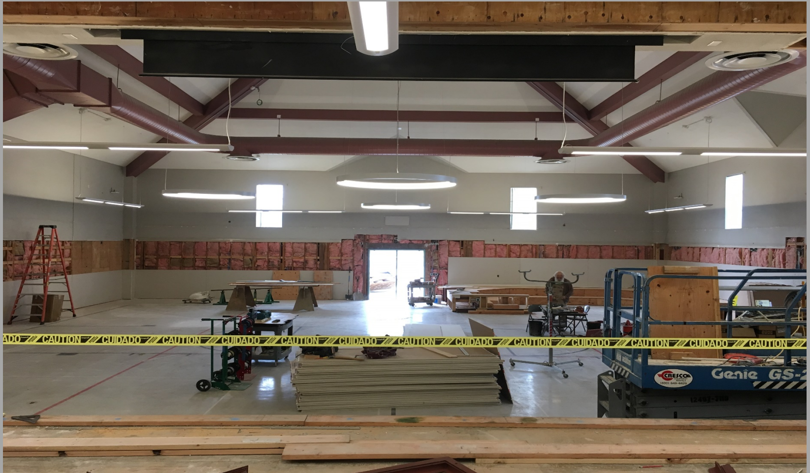
View of South Wall of New Library, from Computer Lab., @ Building E
