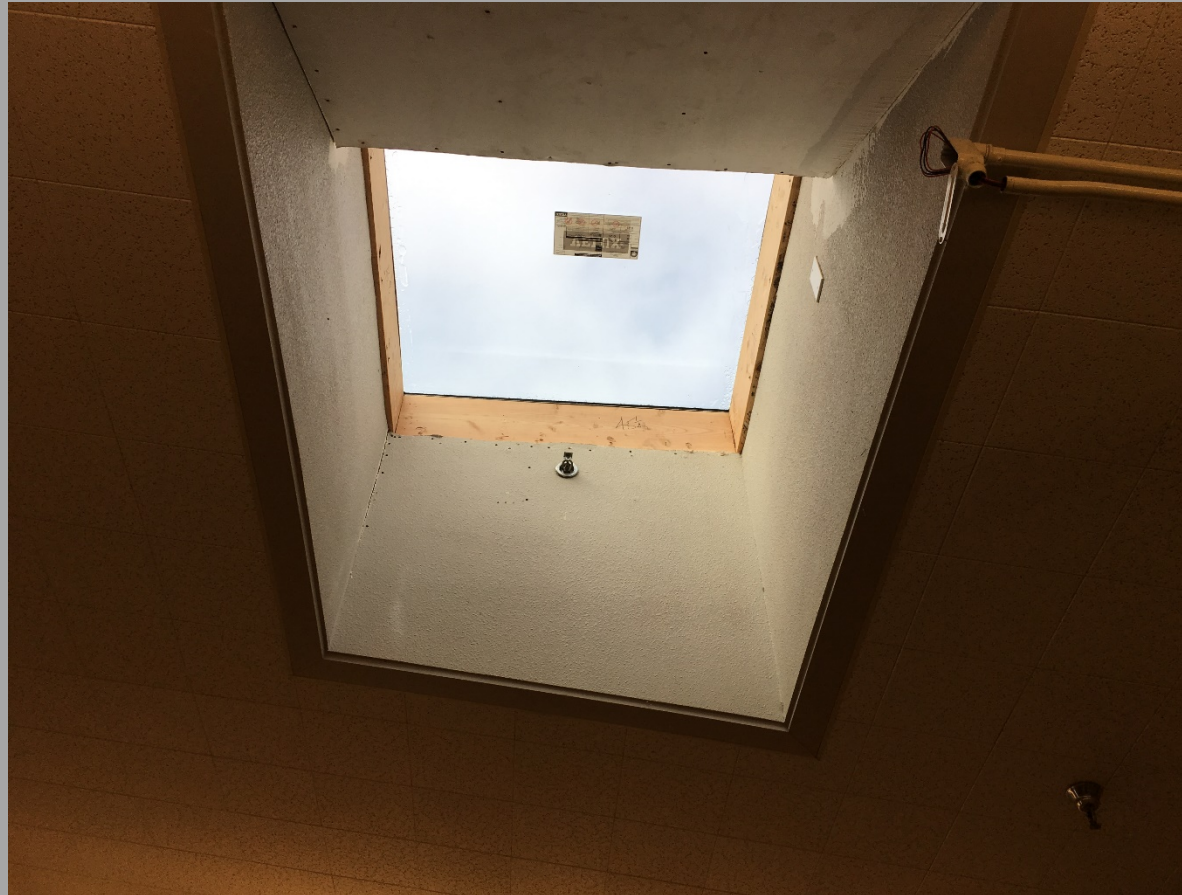
View of One of the New Skylights Above the Computer Lab., @ Building E
