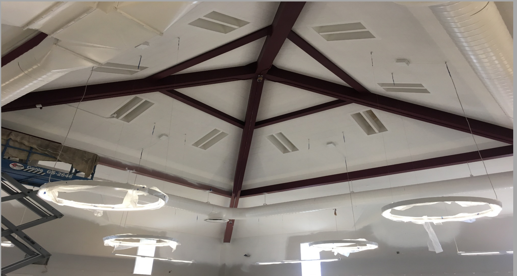
View of Modernization Work @ Building E - New Paint Colors on Ductwork, Beams and Ceiling
