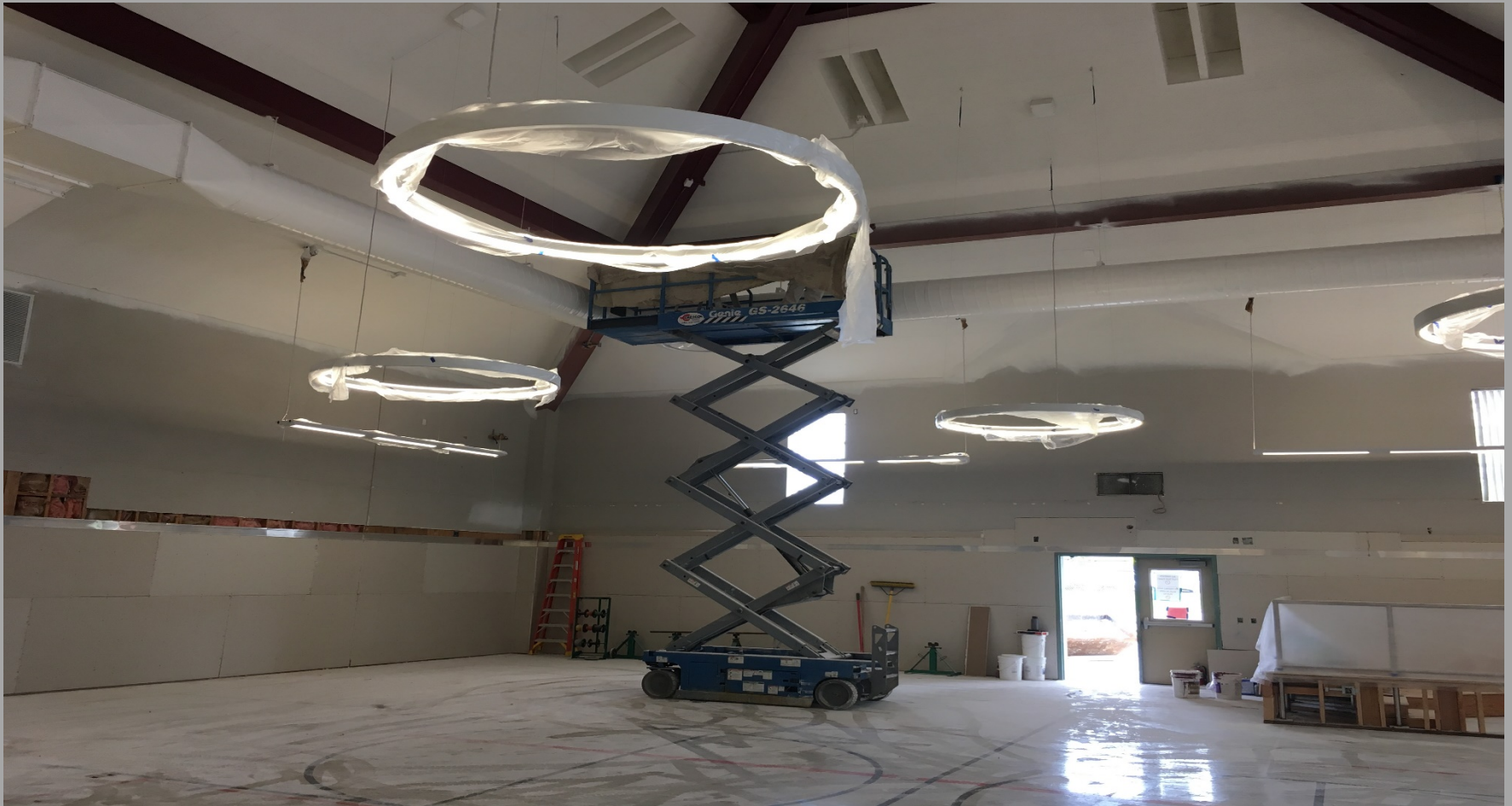
View of Modernization Work @ Building E - Looking Southeast toward Book Shelves Location
