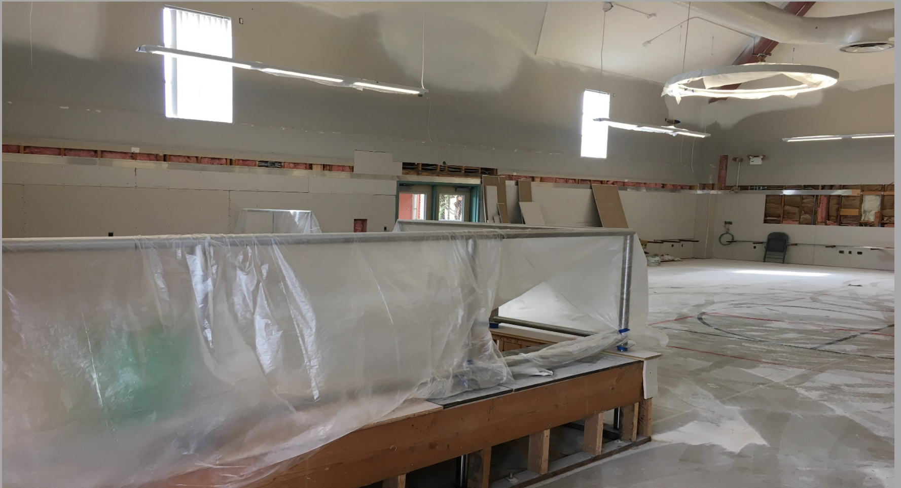
View of Modernization Work @ Building E - Looking Northwest toward Check-Out Counter Location
