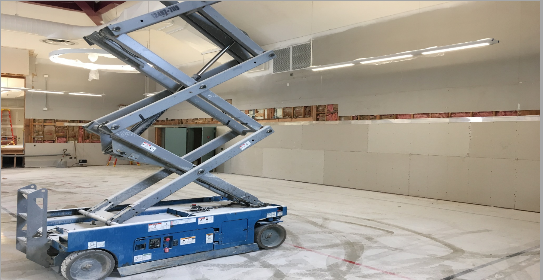
View of Modernization Work @ Building E – Looking Northeast toward Hallway & Book Storage Room
