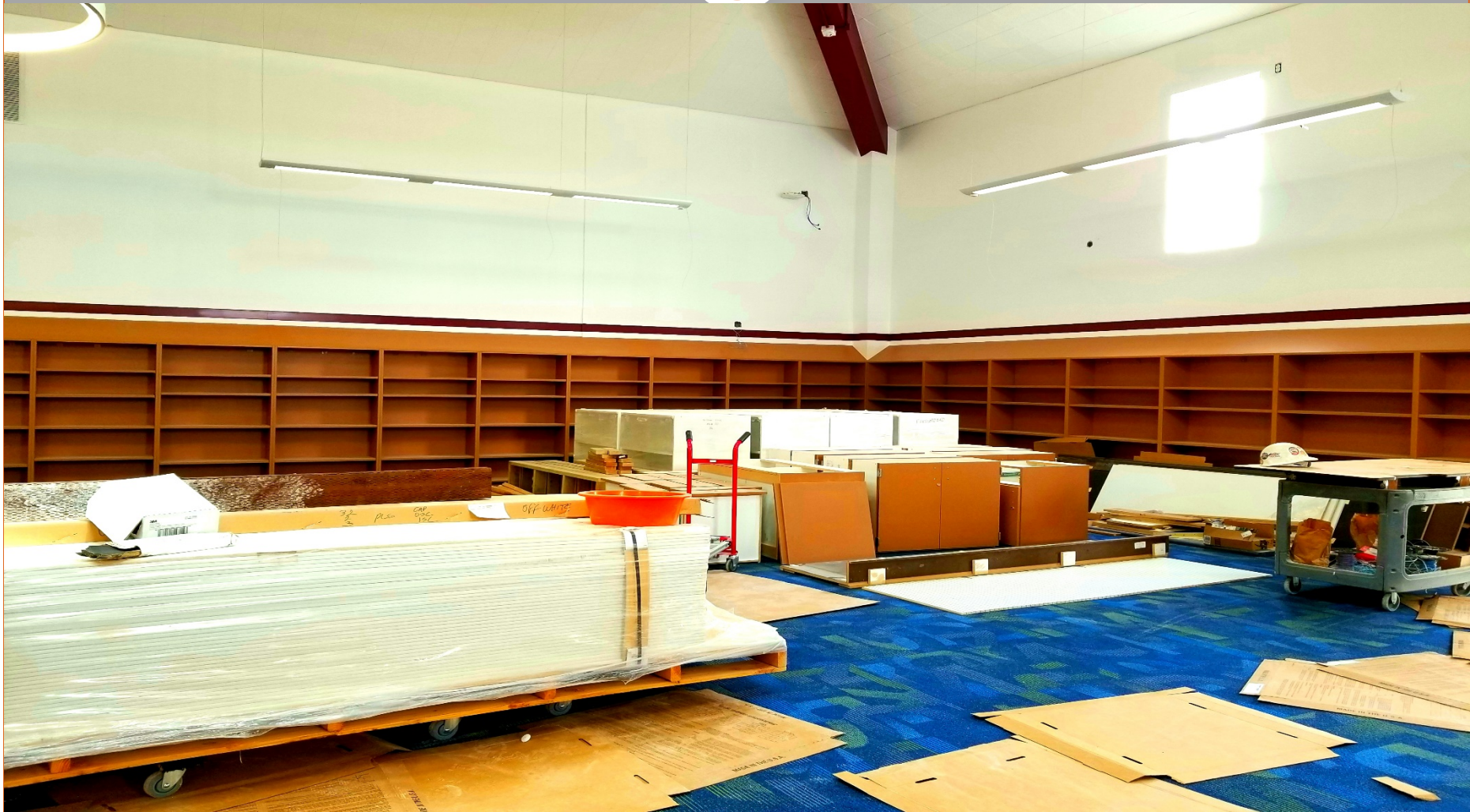
View of South and East Wall of New Library from Computer Lab., @ Building E.
