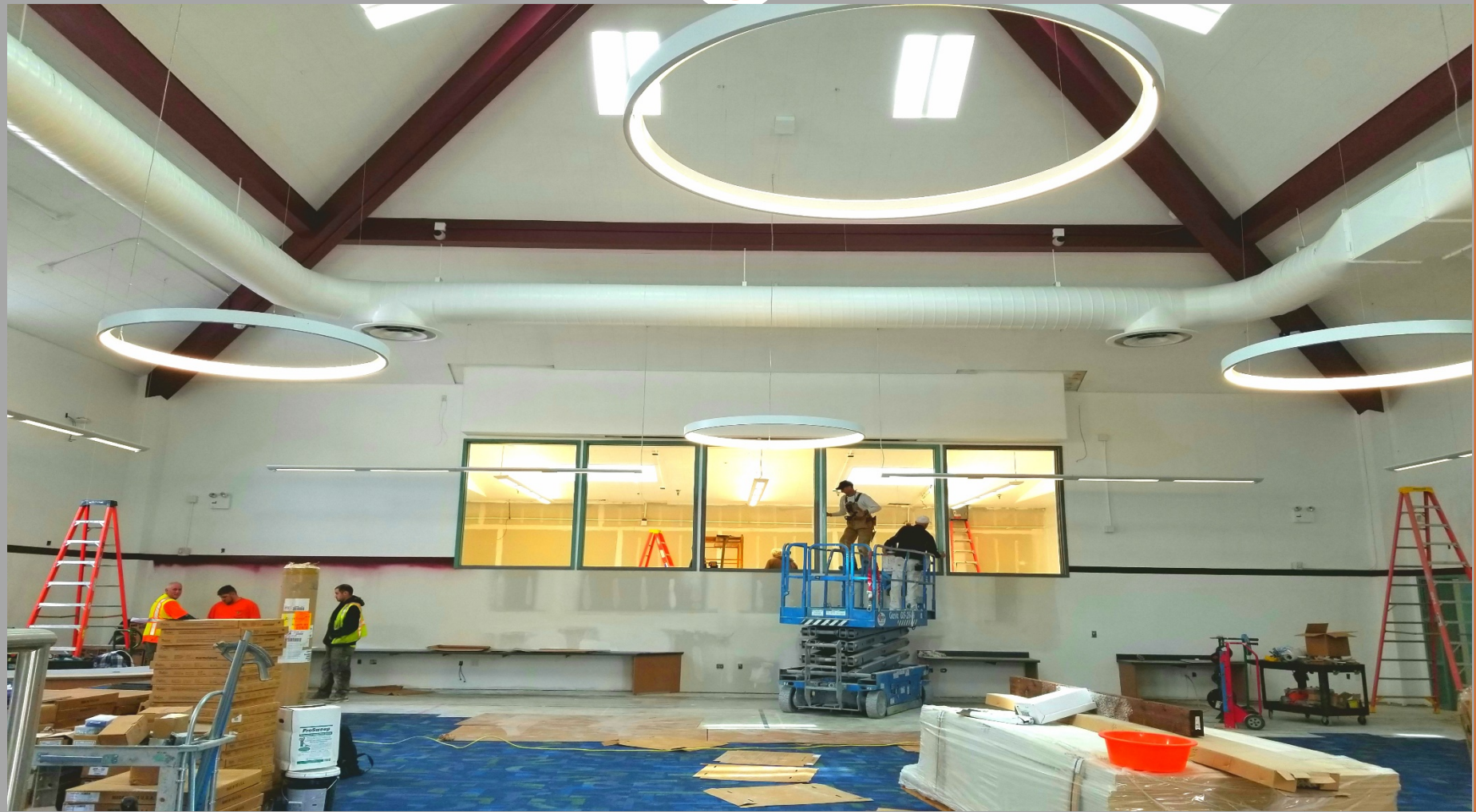
View of Modernization Work @ Building E - Looking North toward Computer Lab. Window wall had been framed & sheetrock was installed.
