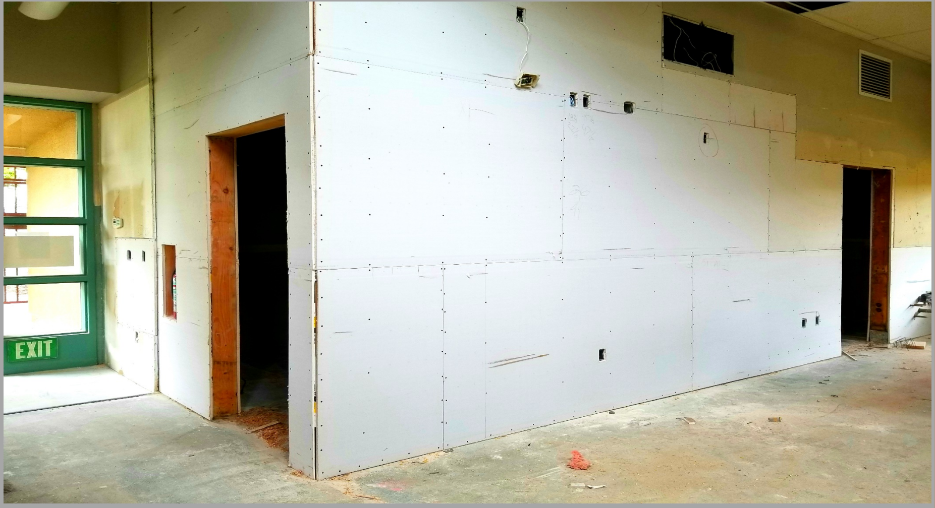
Viewing the Old Library @ Building D - converted offices by framing in the wall.
