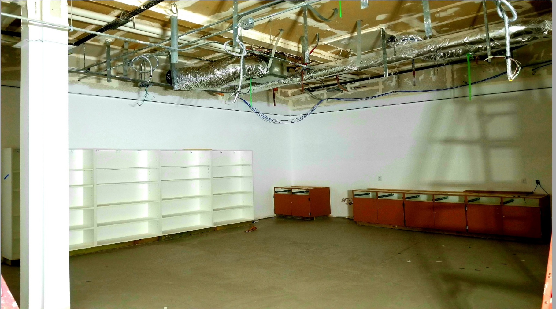
View of Modernization Work Inside of New Book Storage Room @ Building E. Partial cabinets were installed; flooring has been leveled
