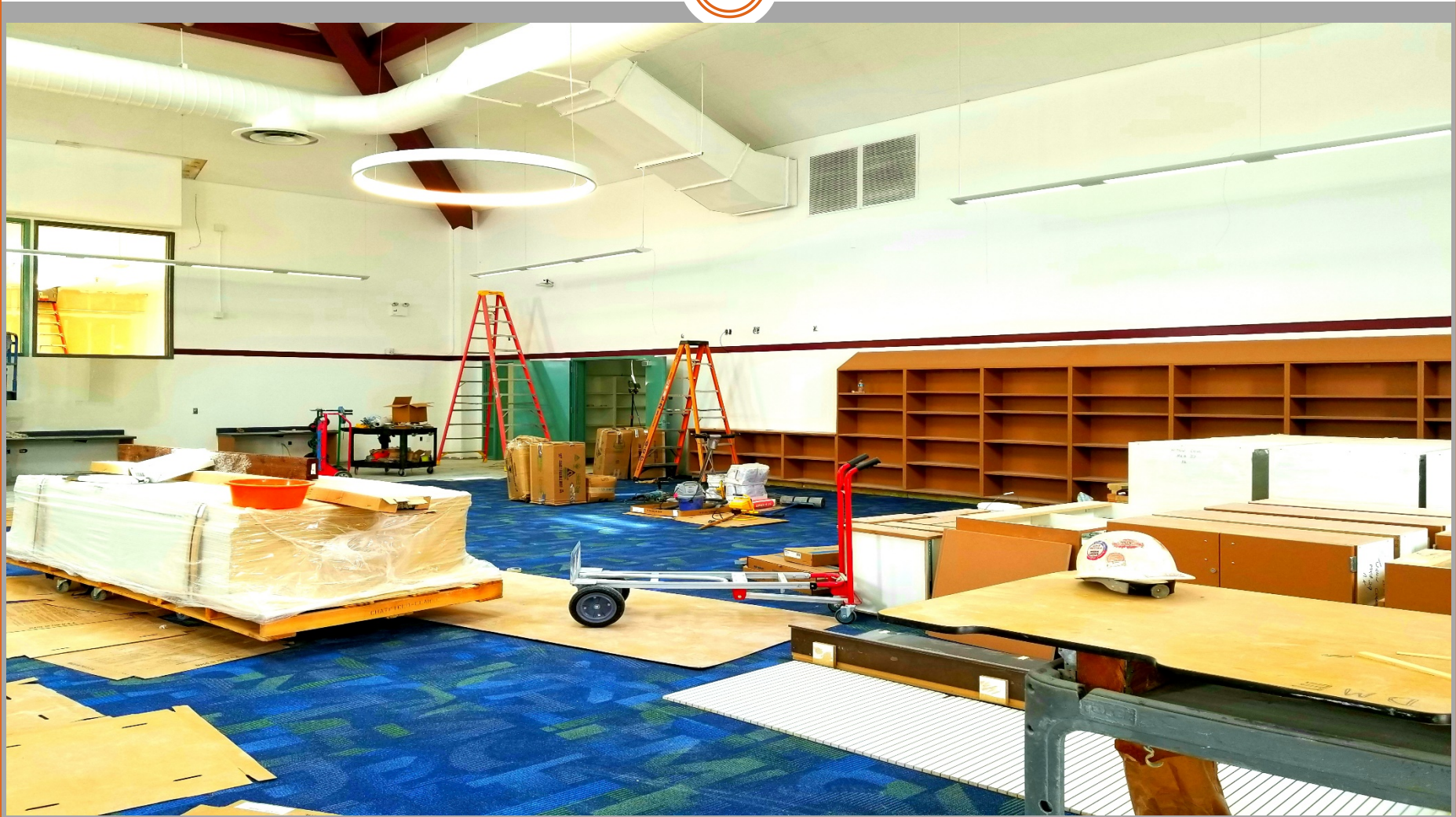
View of Modernization Work @ Building E - Looking Northeast toward Hallway & Book Storage Room. Shelves were installed.
