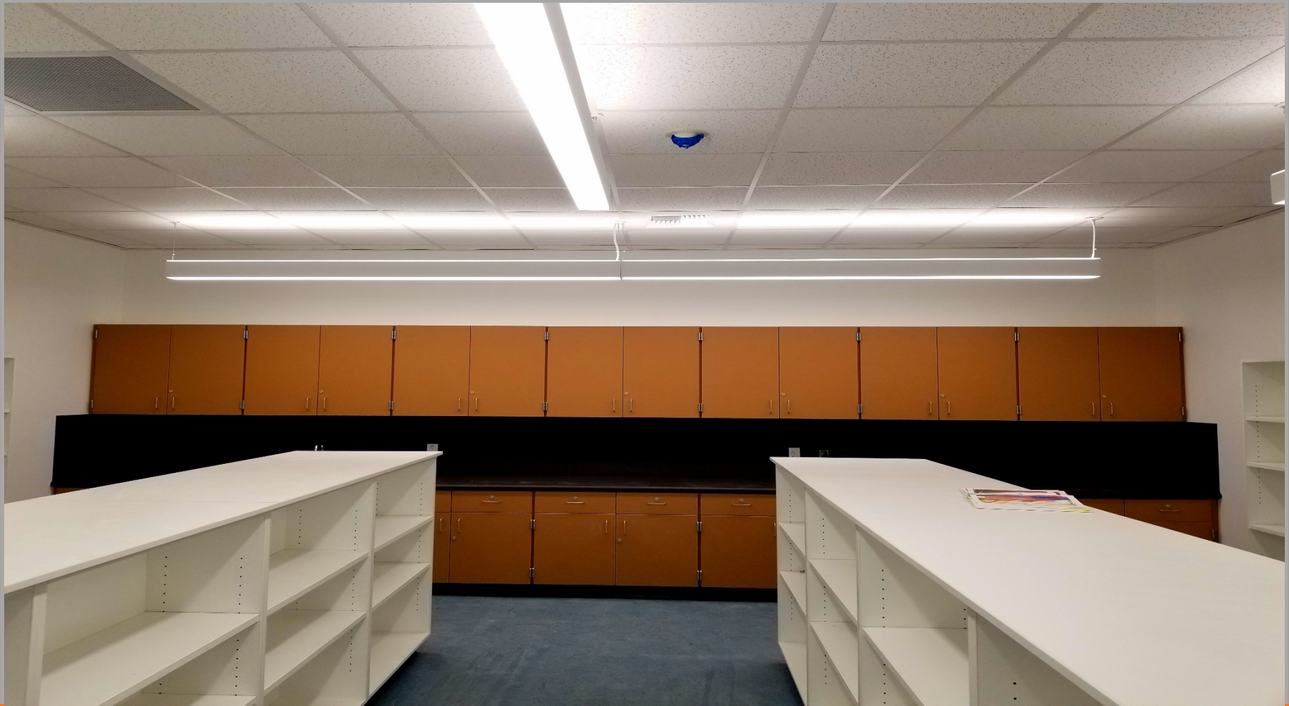
Inside of New Book Storage Room @ Building E – Different angle. Room nearly completed.
