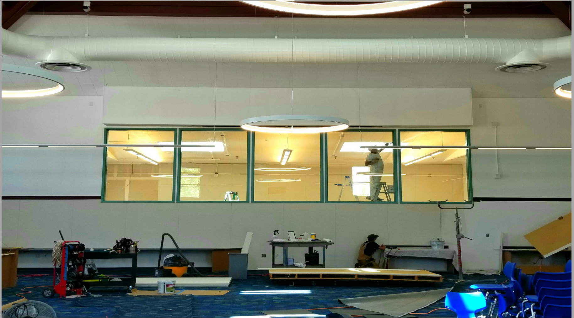
View of Modernization Work @ Building E - Looking North toward Computer Lab. Window glass has been installed.
