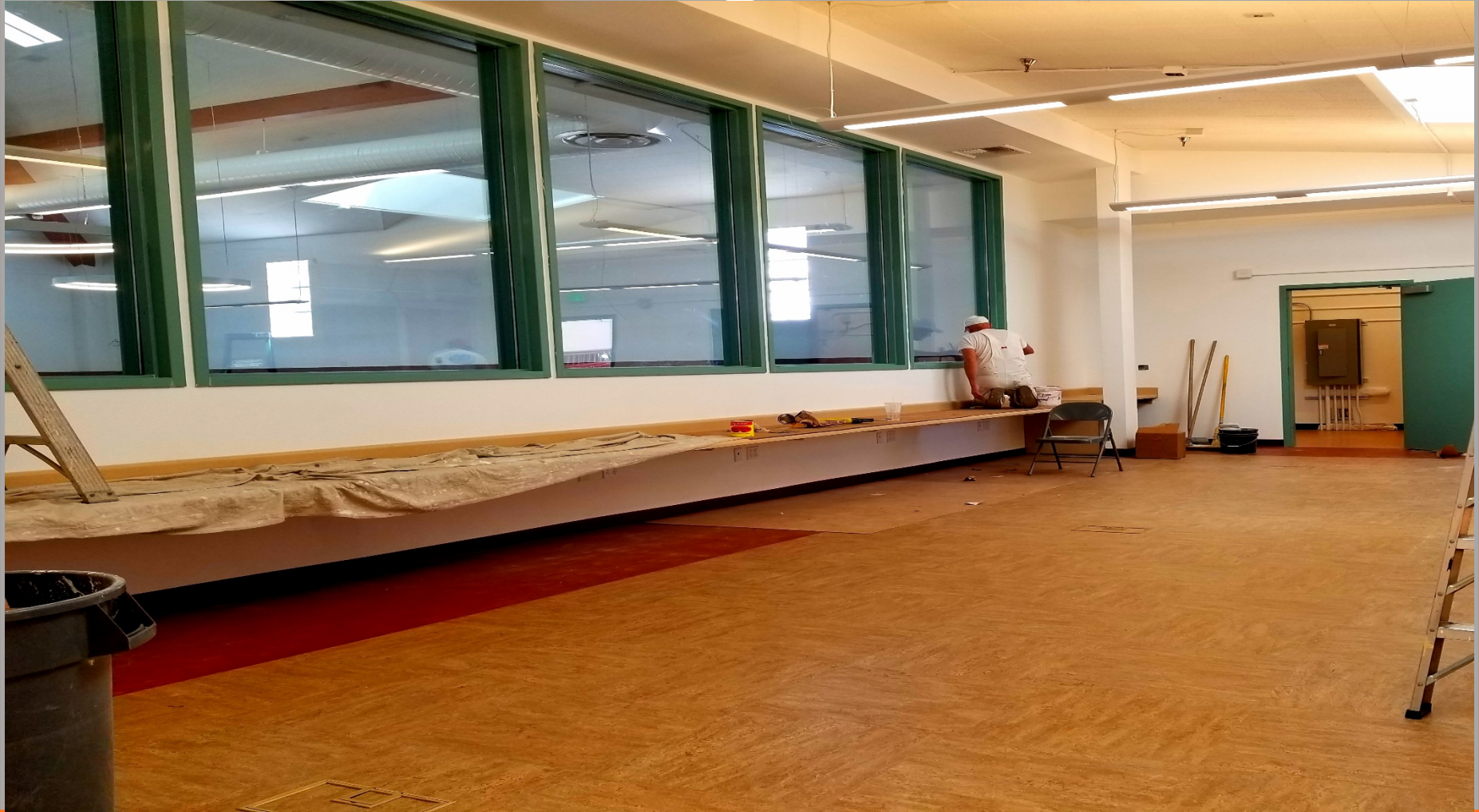
Building E - Viewing the Computer Lab nearing completion. Painter, hard at work.
