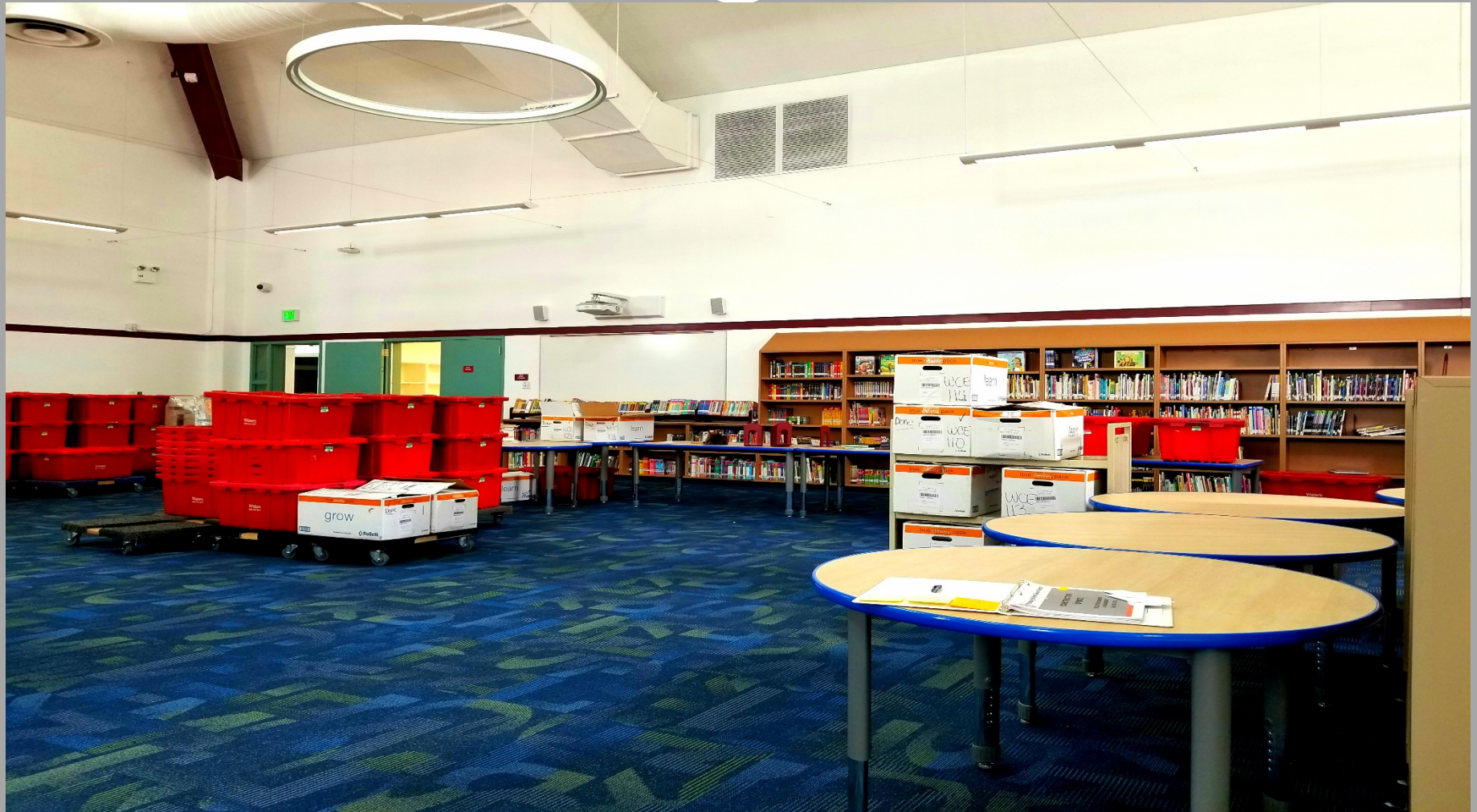
View of Modernization Work @ Building E - Books starting to be placed on the shelves
