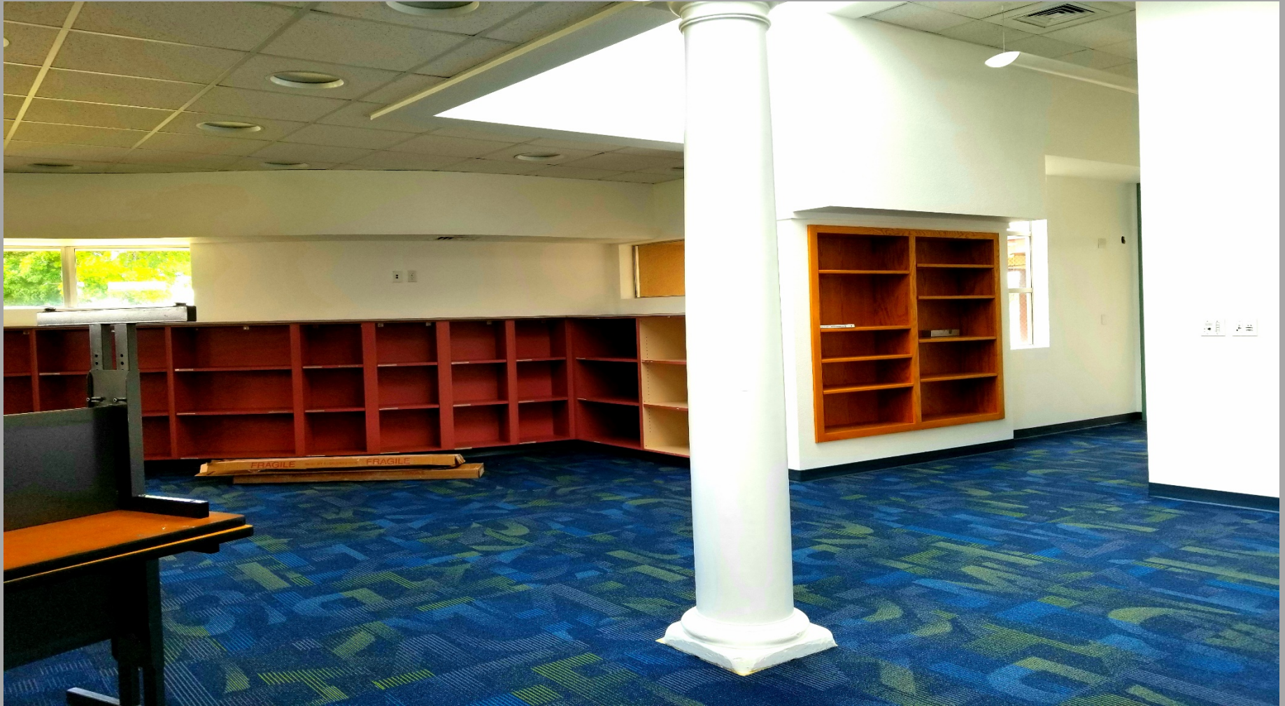
Viewing Building D - carpet and cabinets were installed. Waiting on new interior doors.
