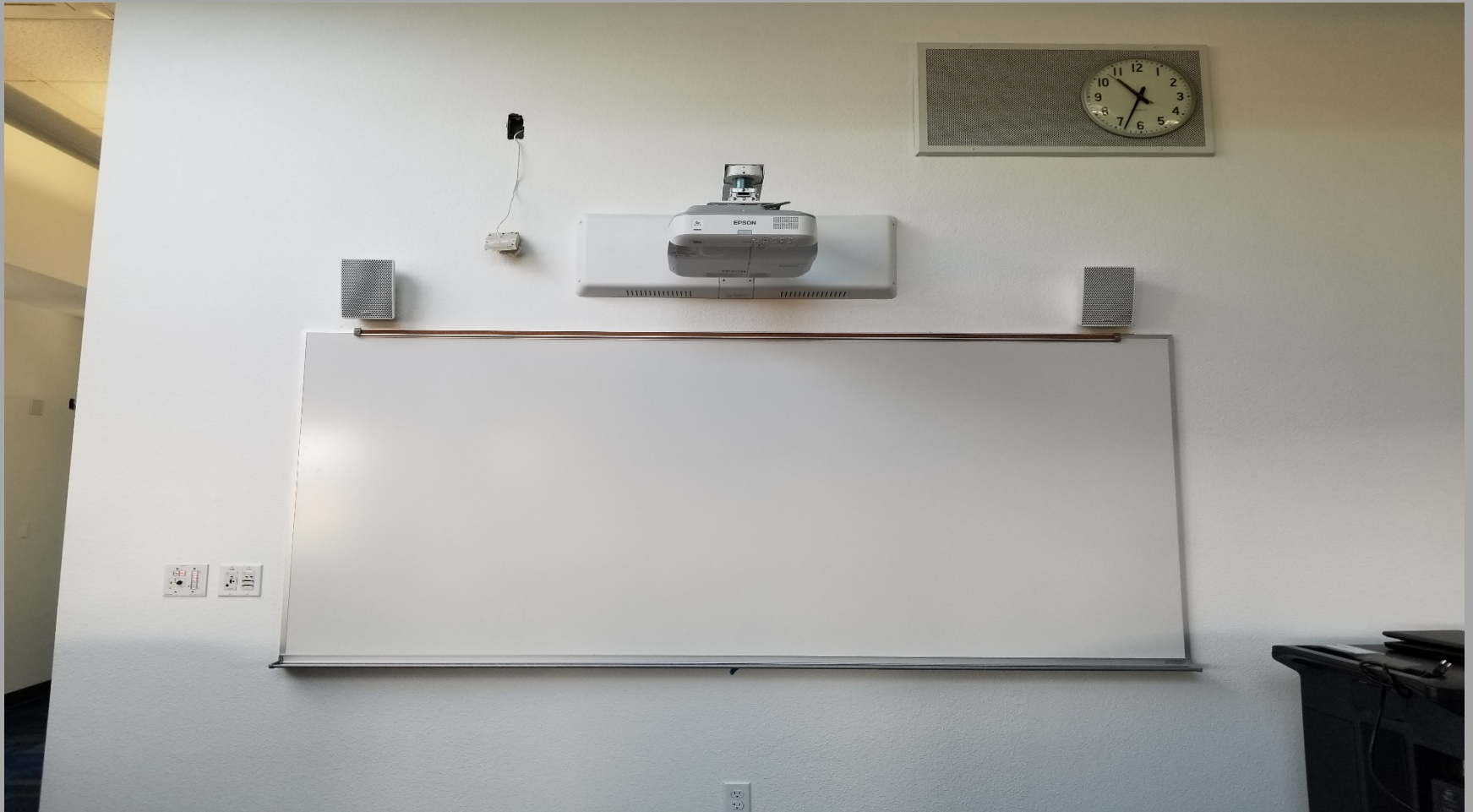
Willow Cove ES Building D - Projector and White Board has been installed
