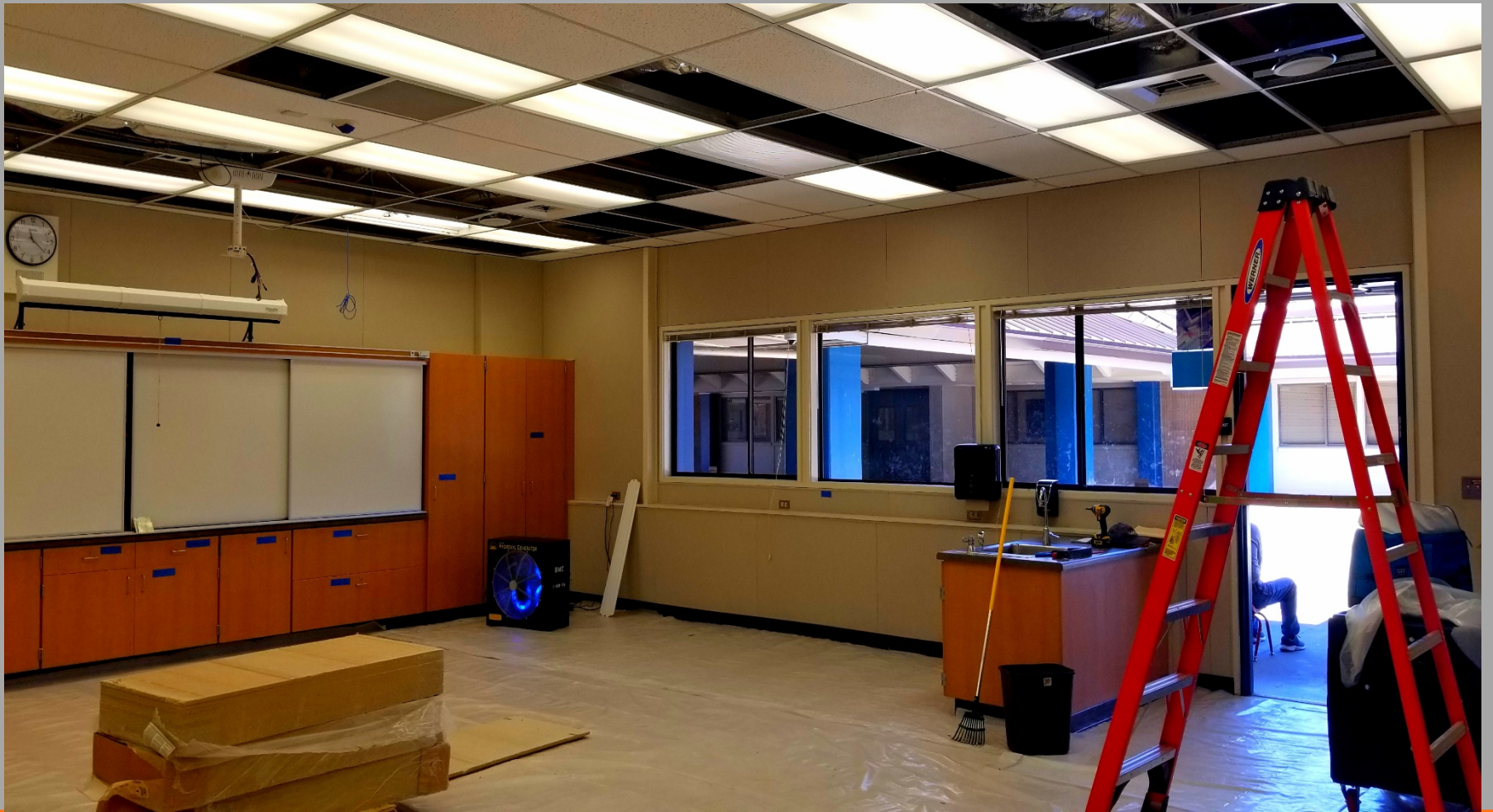
Foothill ES Remediation and Restoration Project caused by fire damage, in progress.
