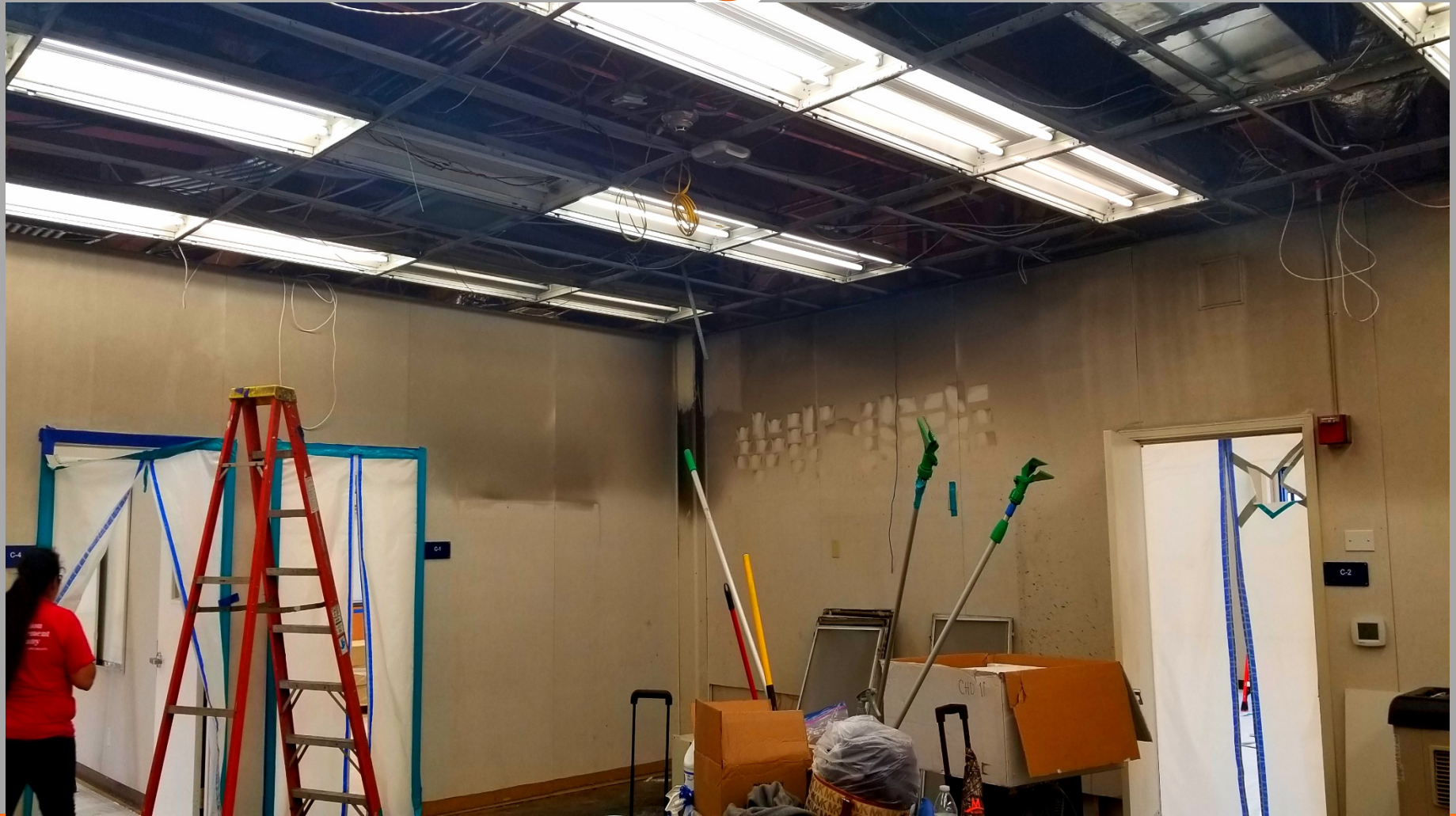
Foothill ES Remediation and Restoration Project caused by fire damage, in progress.
