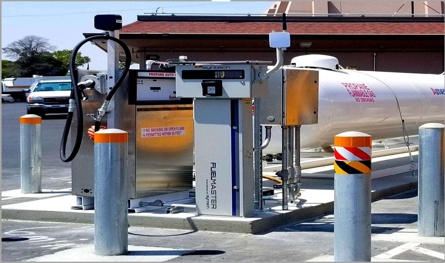
Propane fueling system ready for use.
