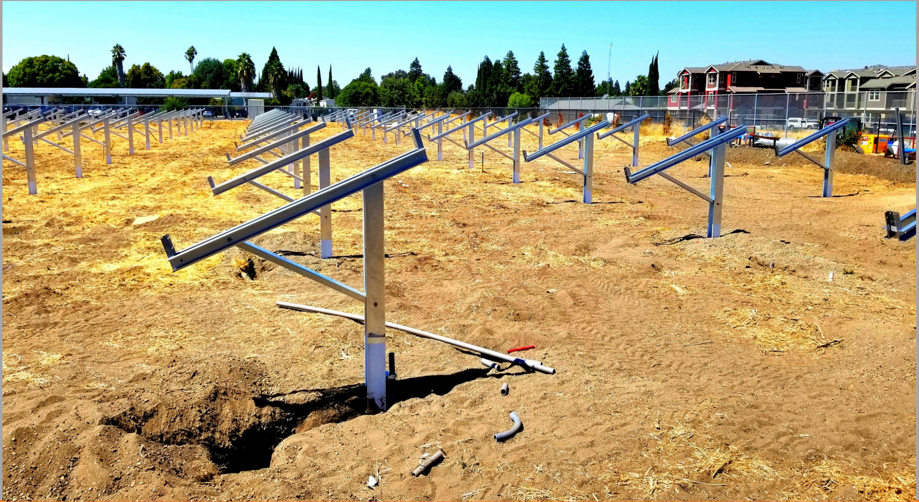
Solar Panels; mounting brackets and posts
