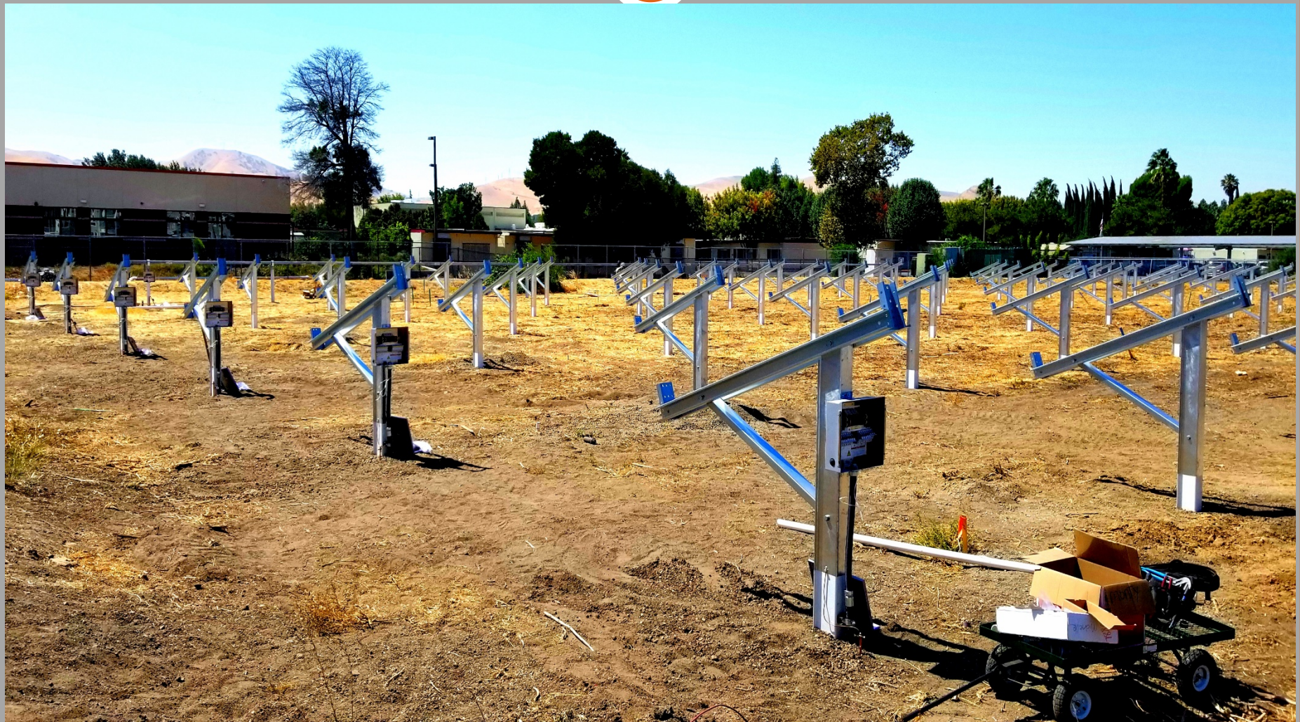
Solar Panels; mounting brackets and posts
