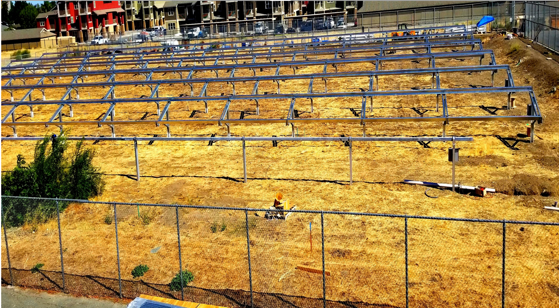
Solar Panels mounting brackets and posts
