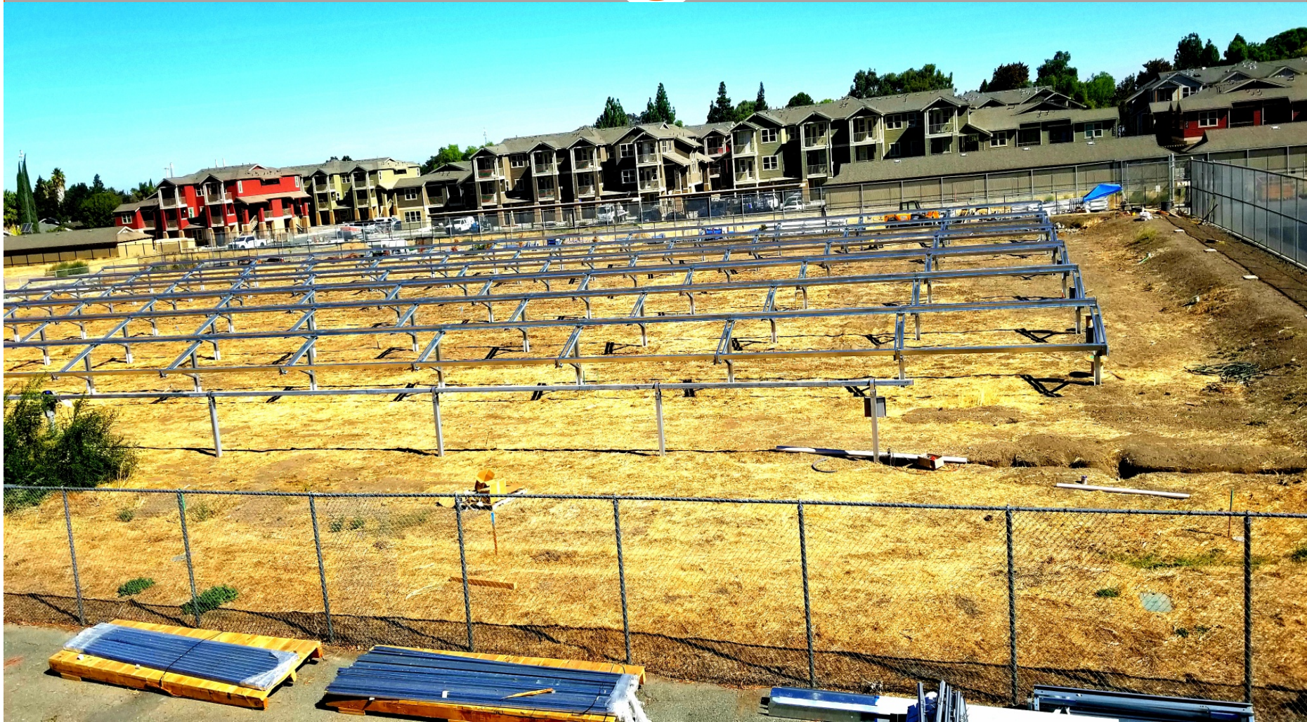
Solar Panels mounting brackets and posts, different angle
