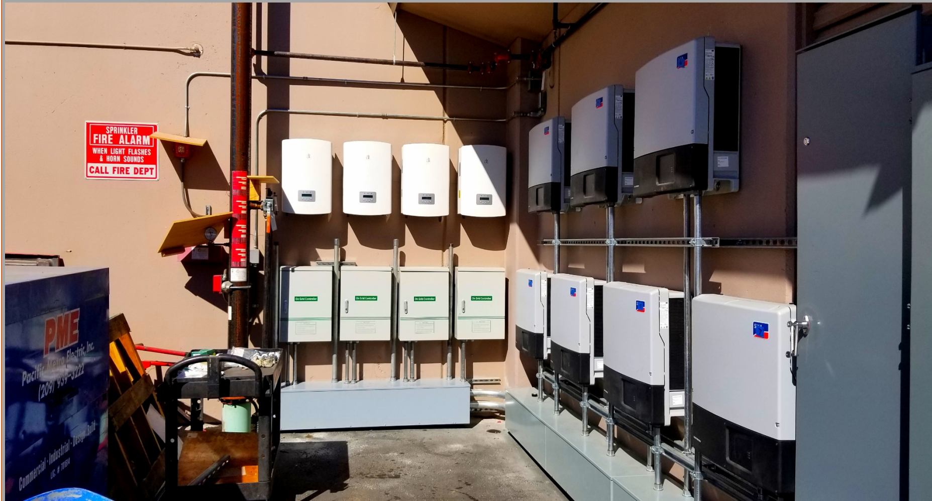
Solar Panel and Wind Turbine inverters at MOT Warehouse
