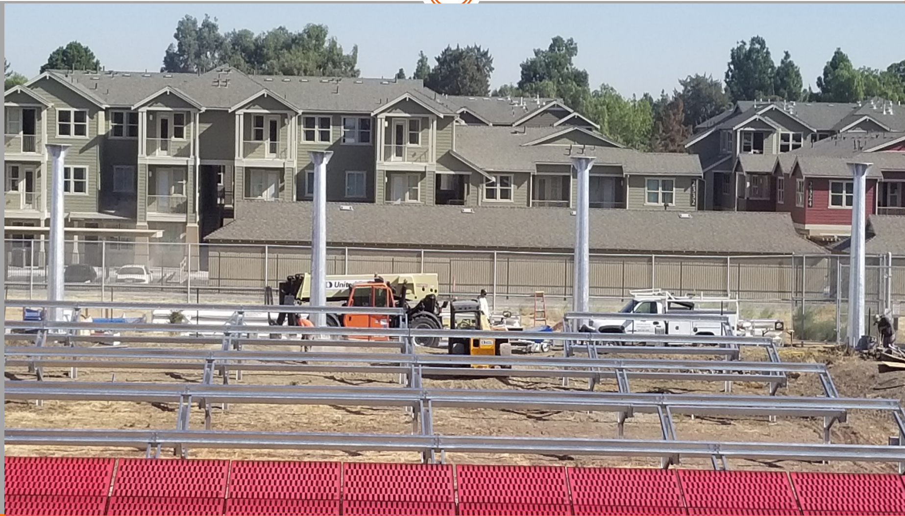
Closer view of solar panel racking & wind turbine supports
