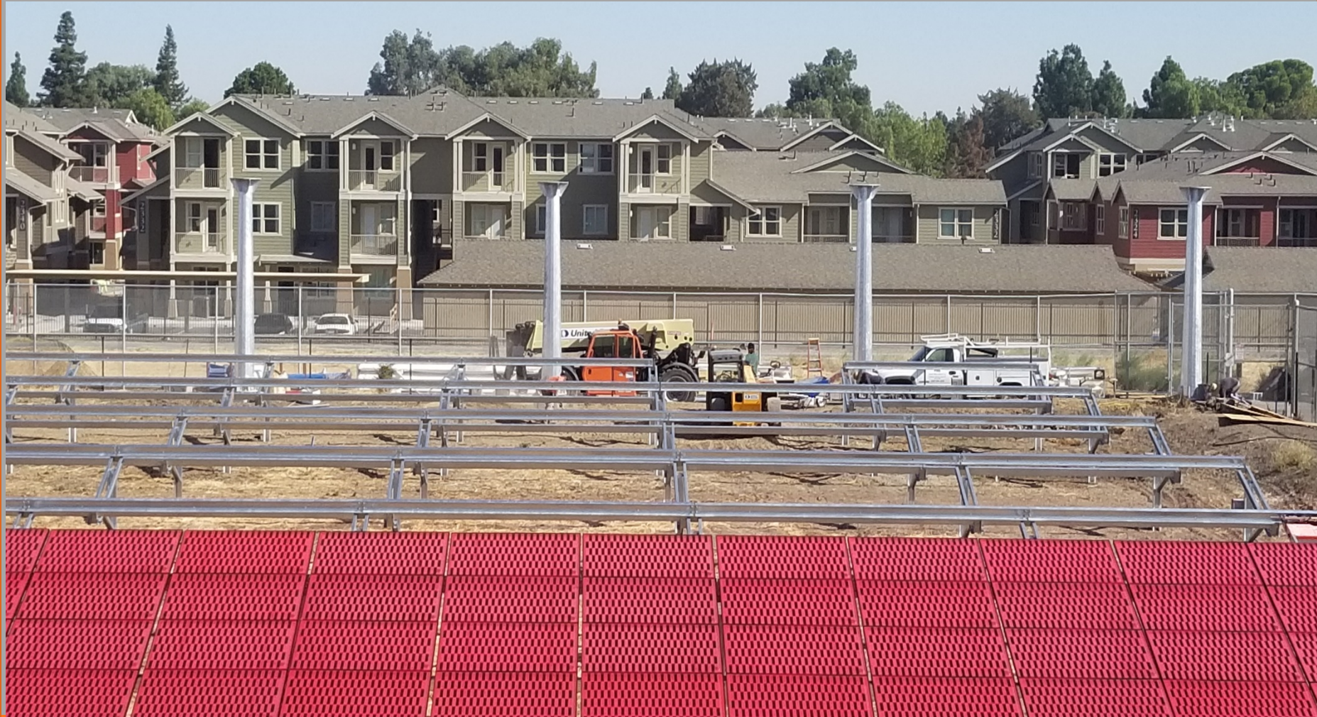
North view, Solar Panel and Wind Turbine inverters at SSSC
