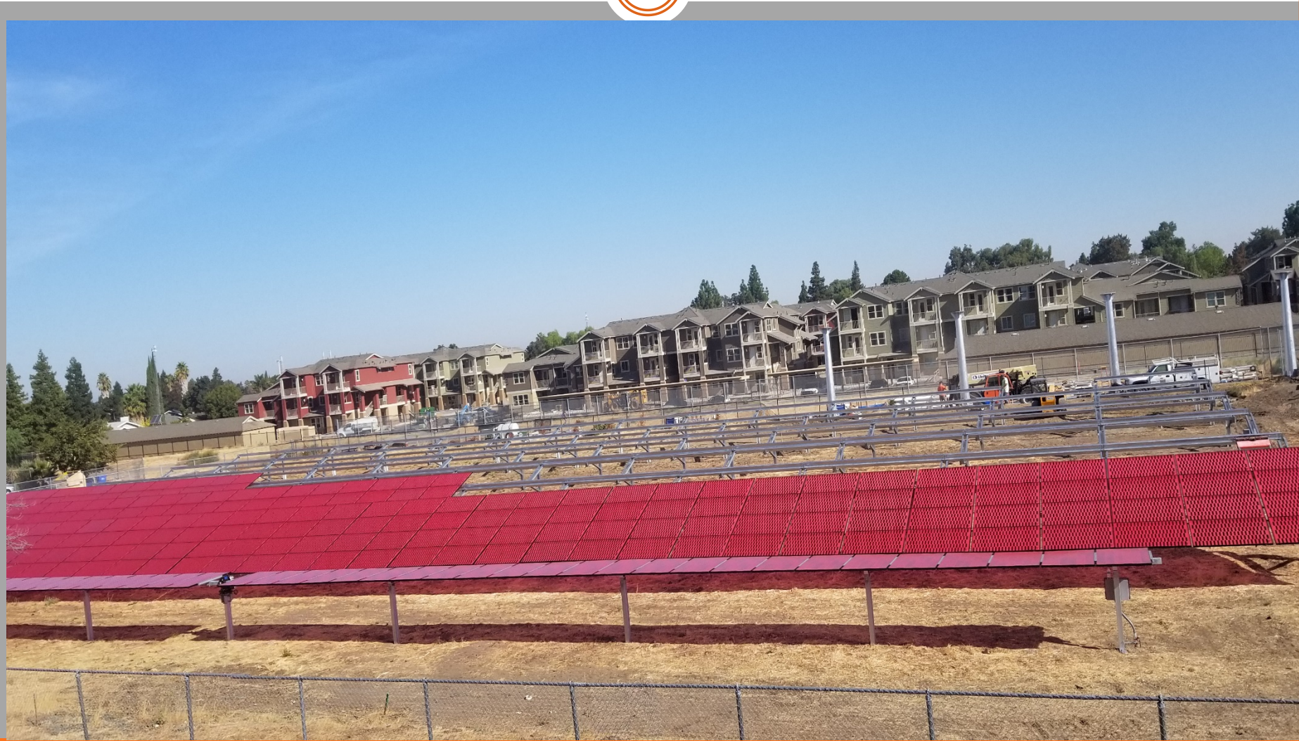
Solar array @ SSSC, Northwest view
