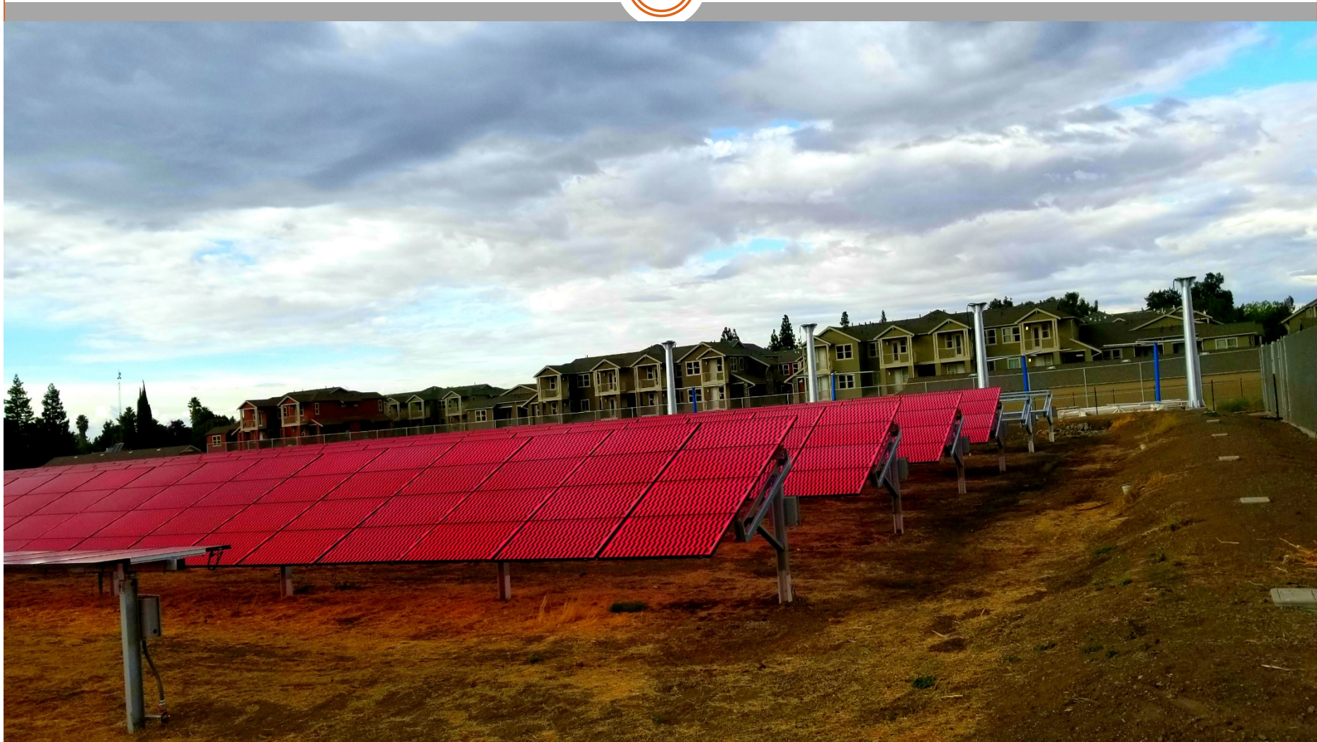
SSSC Solar Panel supports and wind turbine base support poles looking Northwest
