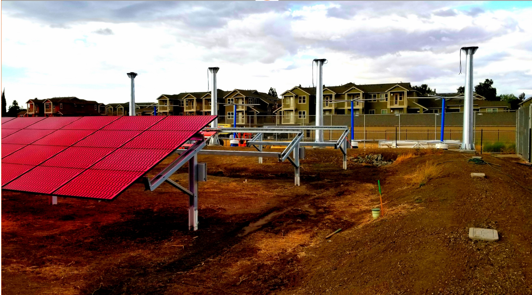
Closer view of solar panel racking & wind turbine supports
