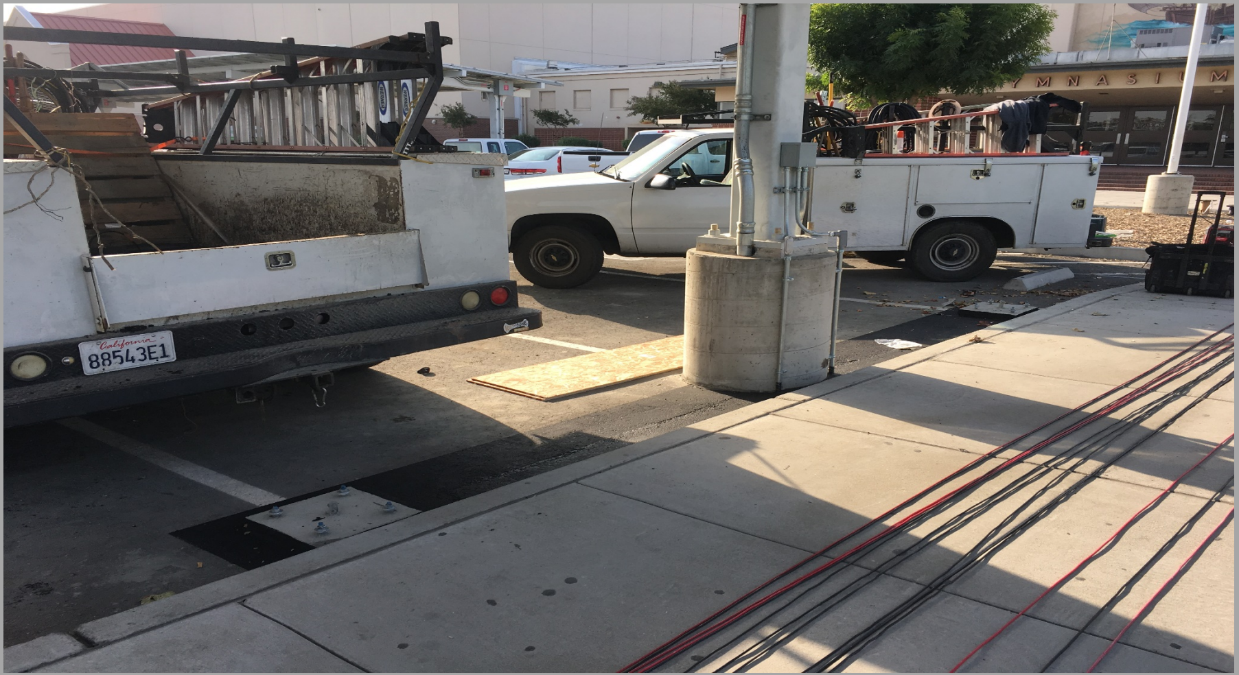
View of Double Dual Head Charging Stations Concrete Pedestals & Wiring for the Charging Stations
