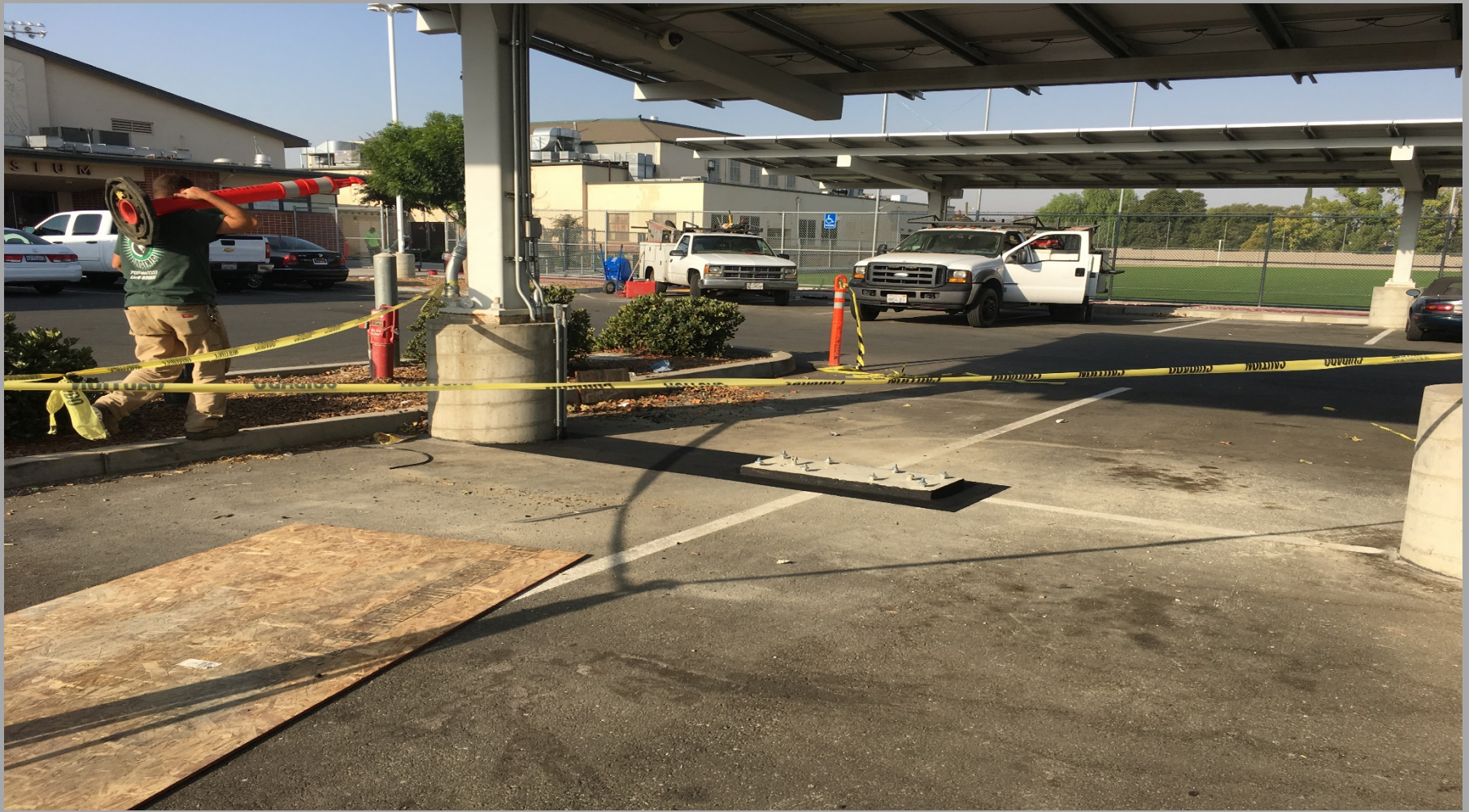
View of Double Dual Head Charging Stations Concrete Pedestals
