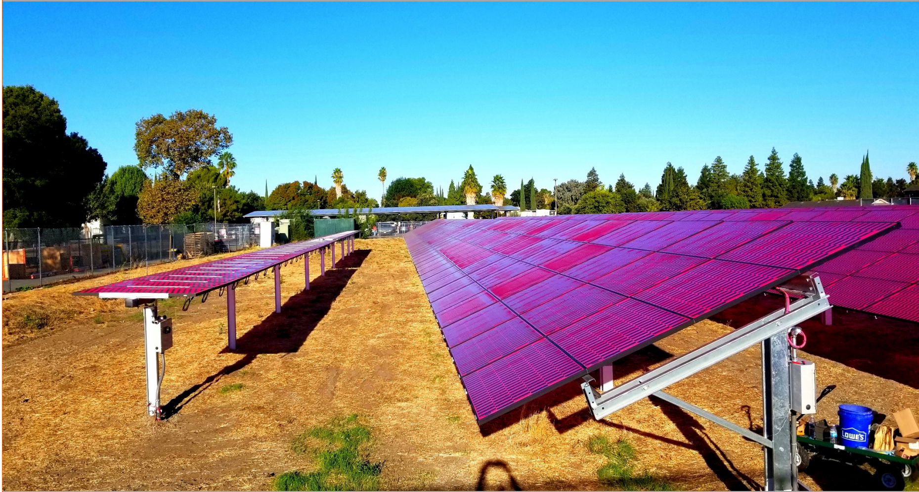
View of Solar/PV Panels from inside of Bioswale
