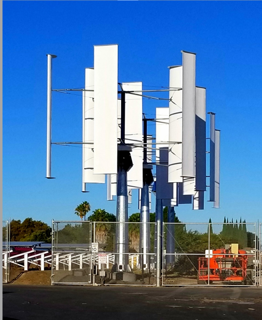
SSSC Wind Turbines
