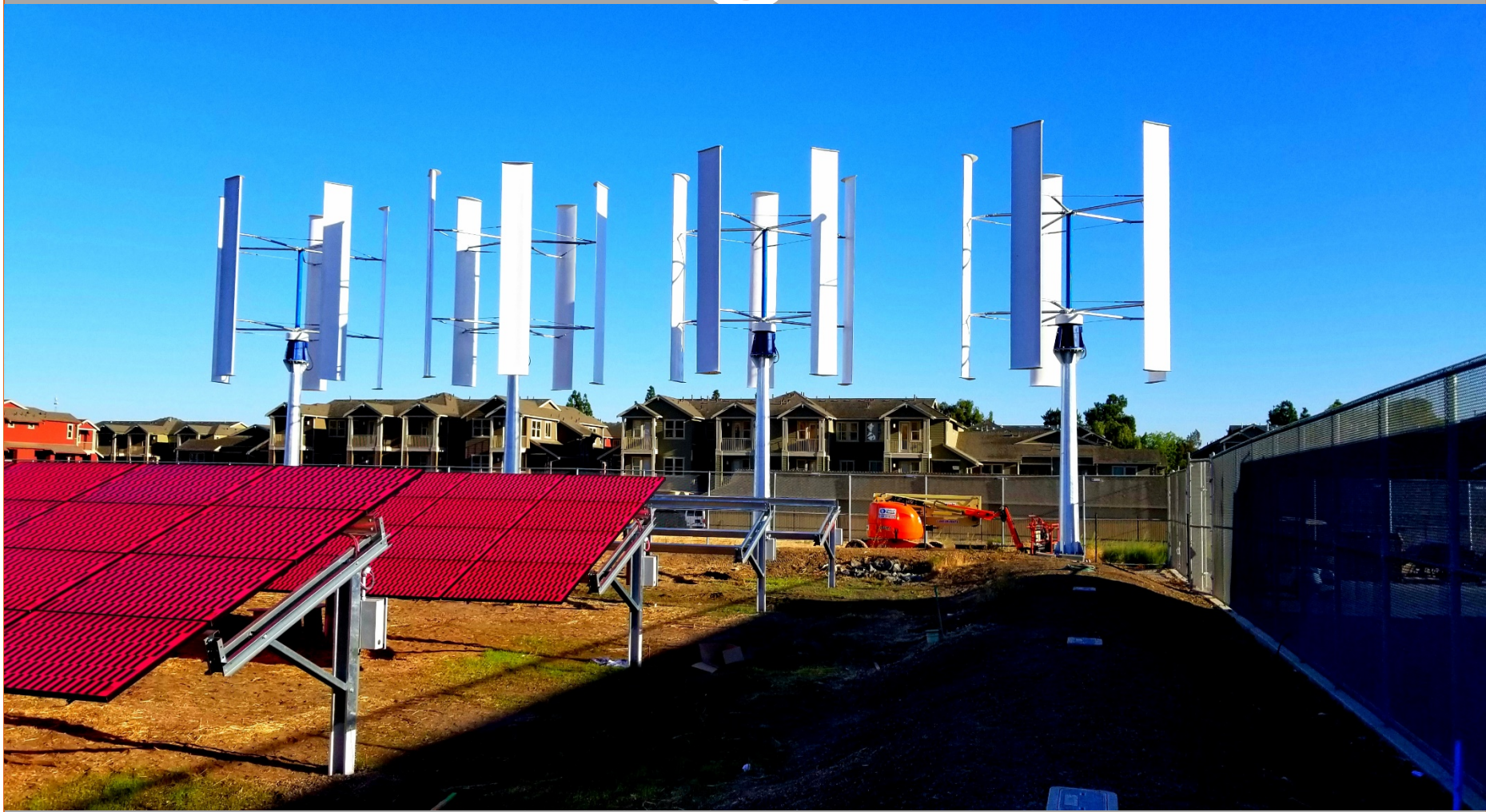
View of Solar/PV Panels & Wind Turbines from inside of Bioswale
