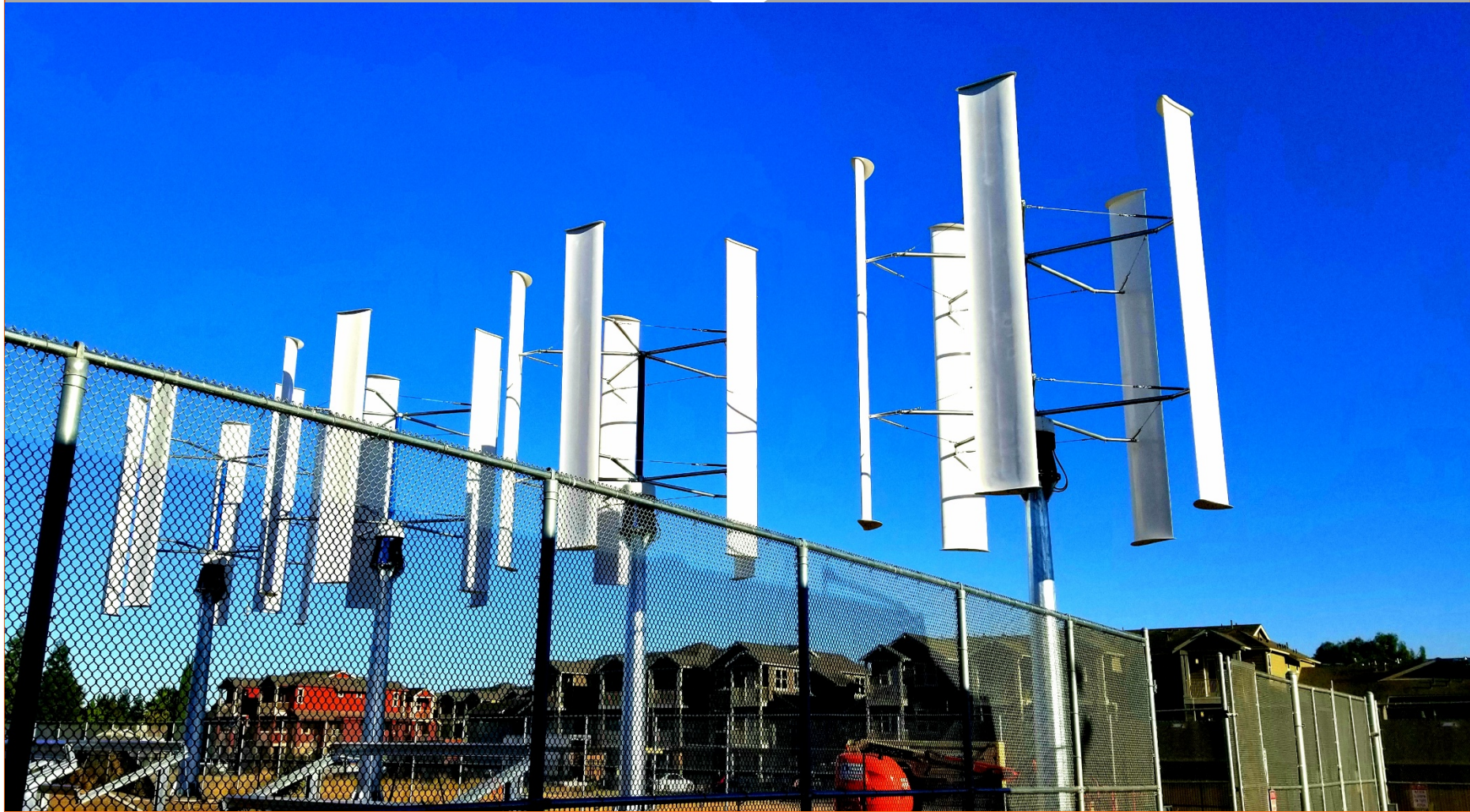
Close-Up View of Wind Turbines
