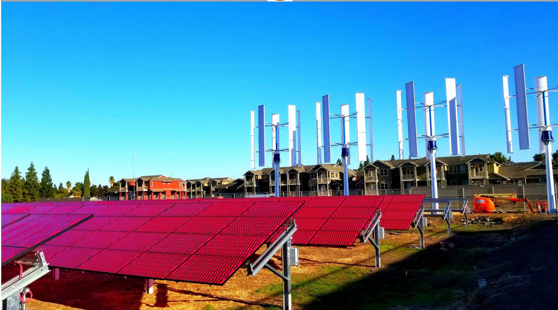
Closer view of Solar/PV Panels & Wind Turbines
