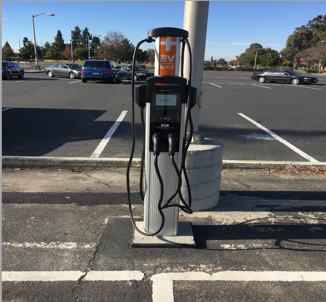
Up-Close View of Completed EV Charging Station – To Be Commissioned
