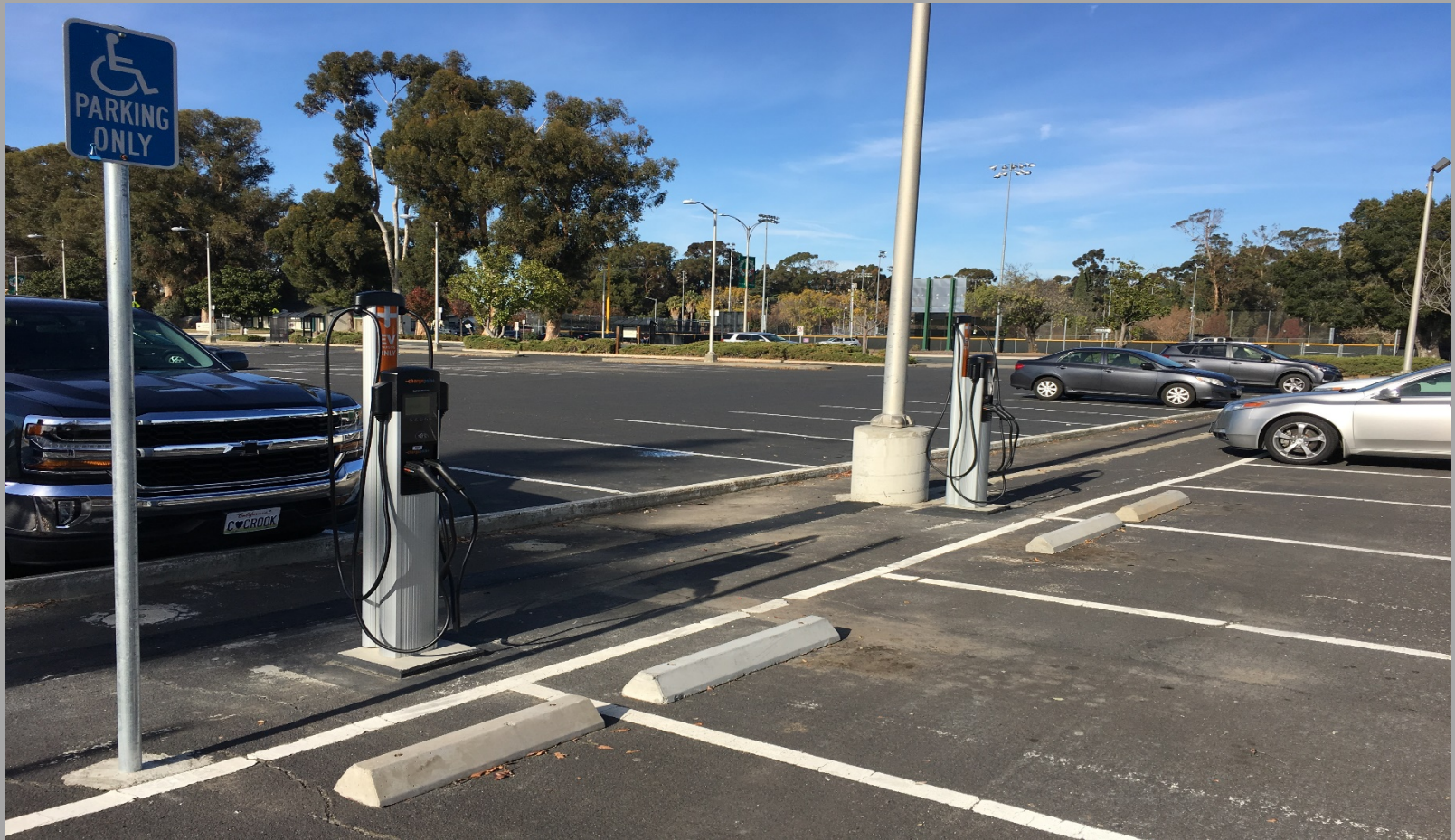
View of Completed EV Charging Stations – To Be Commissioned
