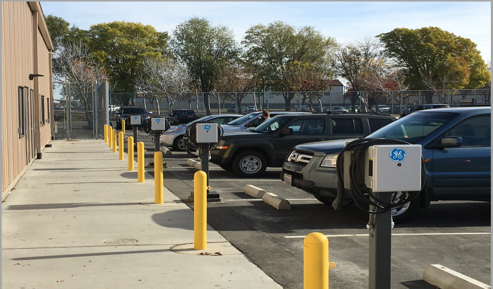
View of Completed & Operating EV Charging Stations
