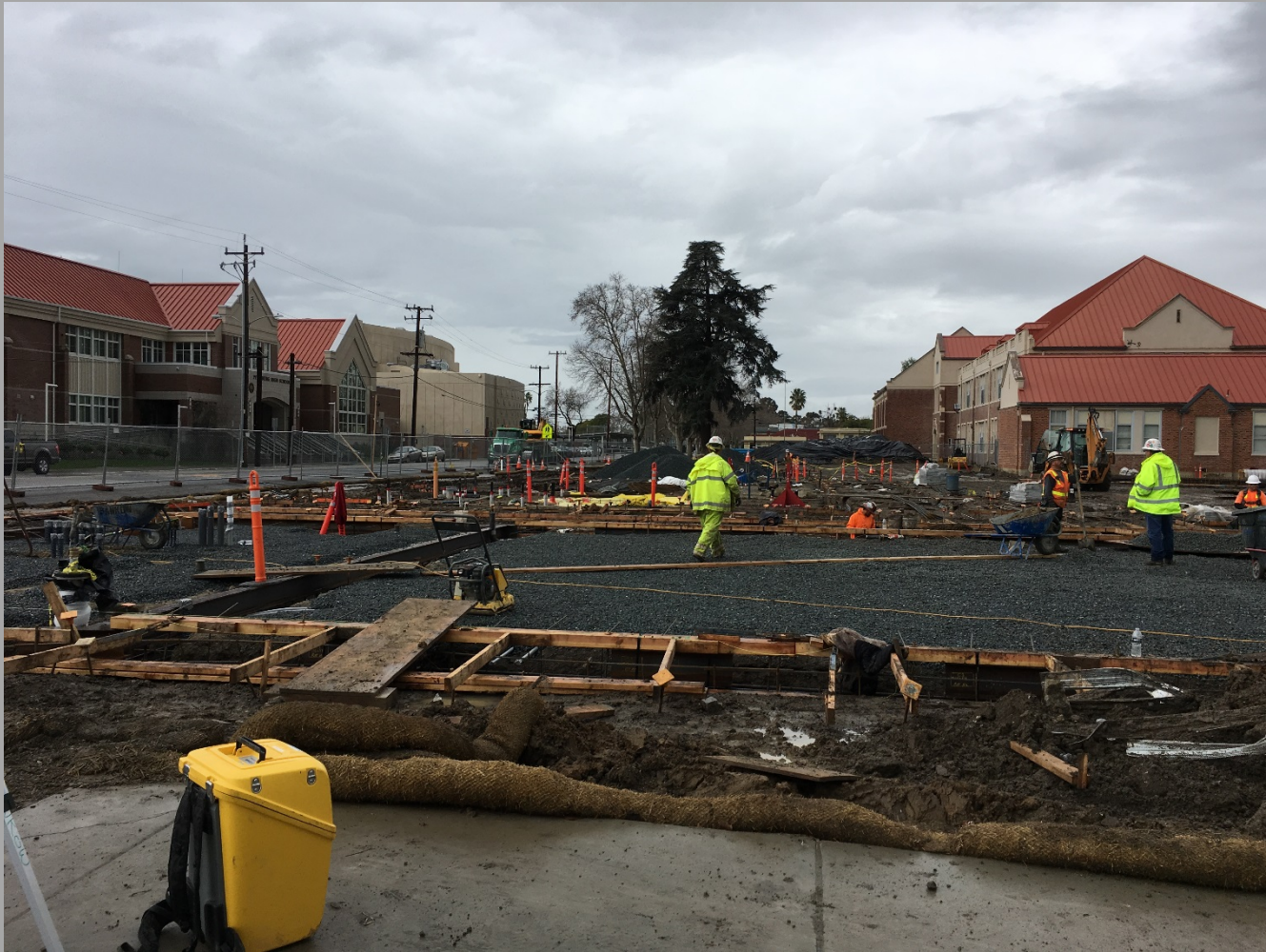
New 8 Classrooms Bldg. (Bldg. N3) Footings & Slab Concrete Pour Preparation Ongoing – Looking West
