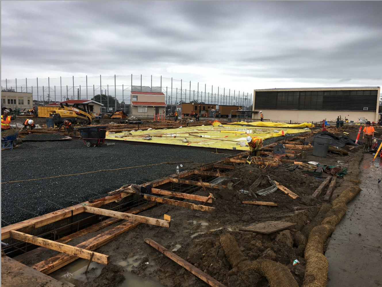
New 10 Classrooms Bldg. (Bldg. N2) Footings & Slab Area Being Readied for Concrete Pour - Looking Northwest
