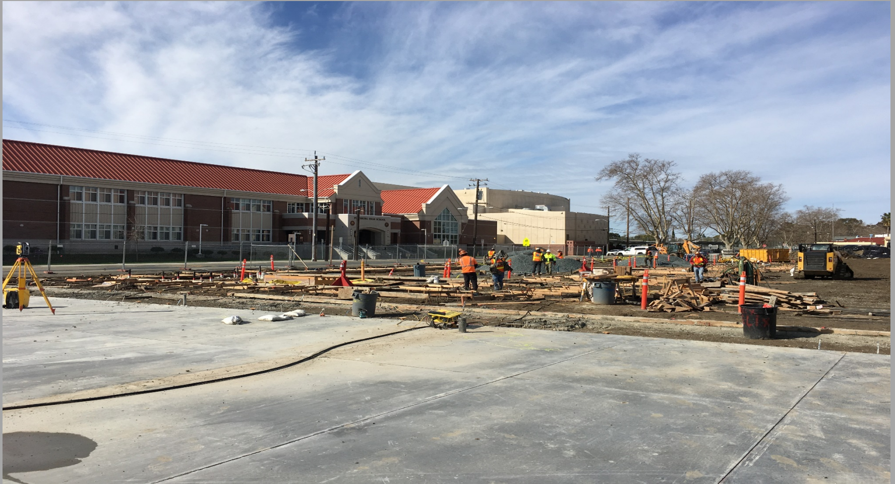
New 8 Classrooms Bldg. (Bldg. N3) Footings & Slab Area Being Readied for Concrete Pour – Looking Southwest
