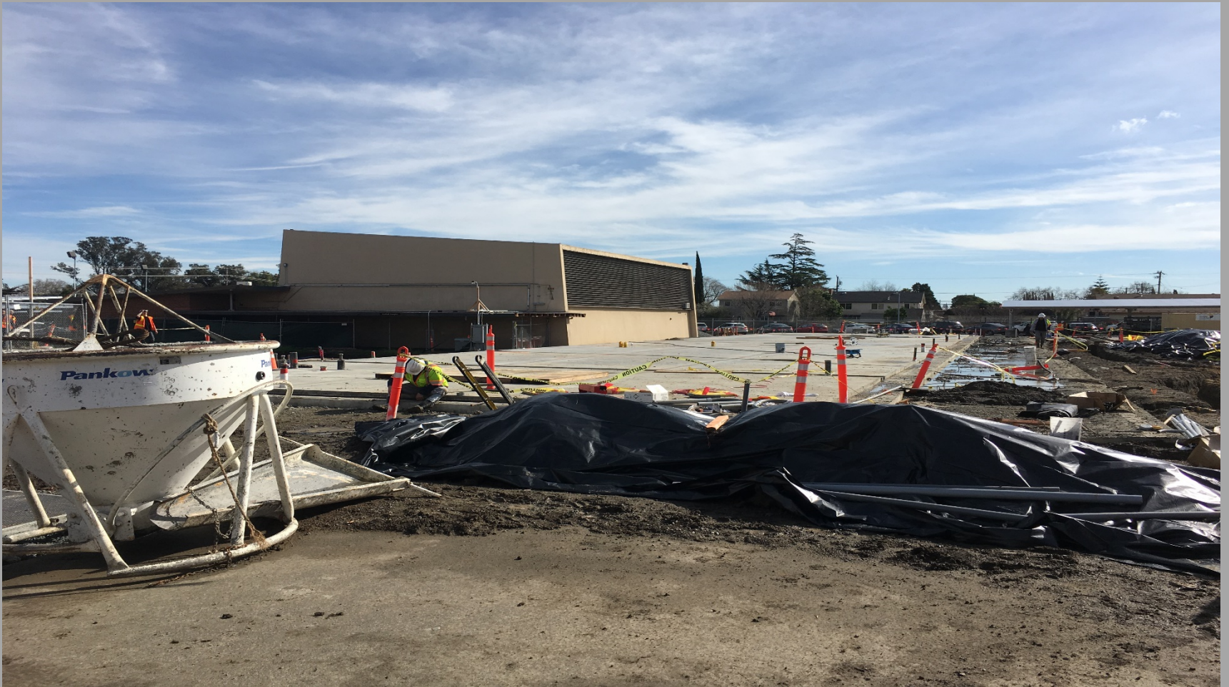
New 12 Classrooms Bldg. (Bldg. N1) Slab Poured & Prepping for Wall Panels- Looking Southeast
