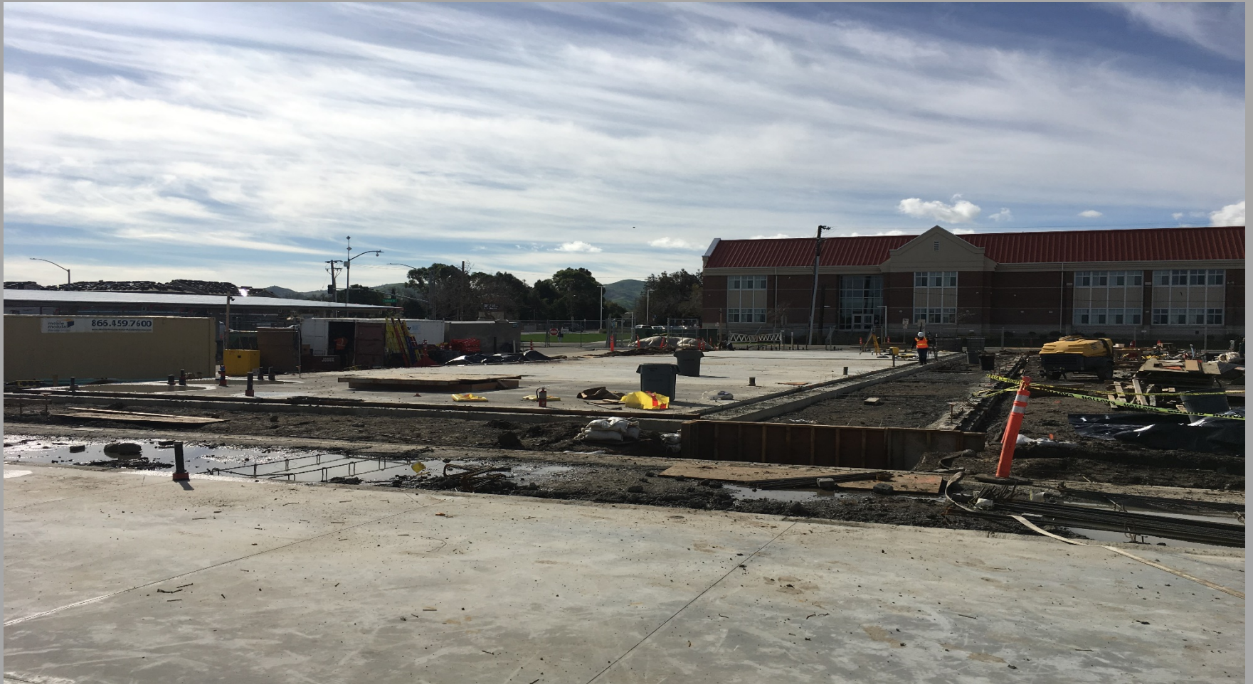
New 10 Classrooms Bldg. (Bldg. N2) Slab Poured & Prepping for Wall Panels – Looking Southeast
