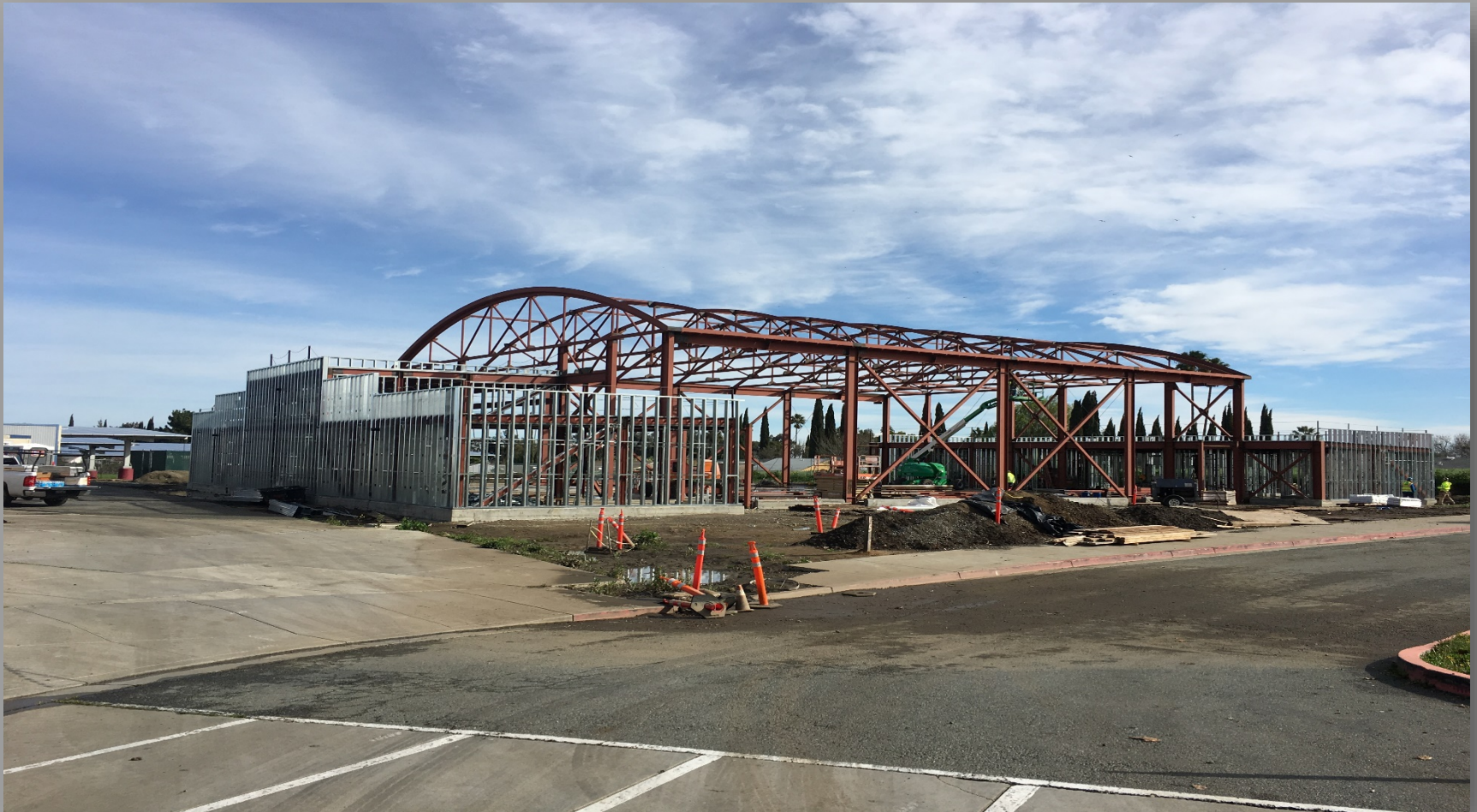
New Gym./MP Bldg. Roof Trusses in place & Exterior Walls Framing Ongoing- Looking Northeast
