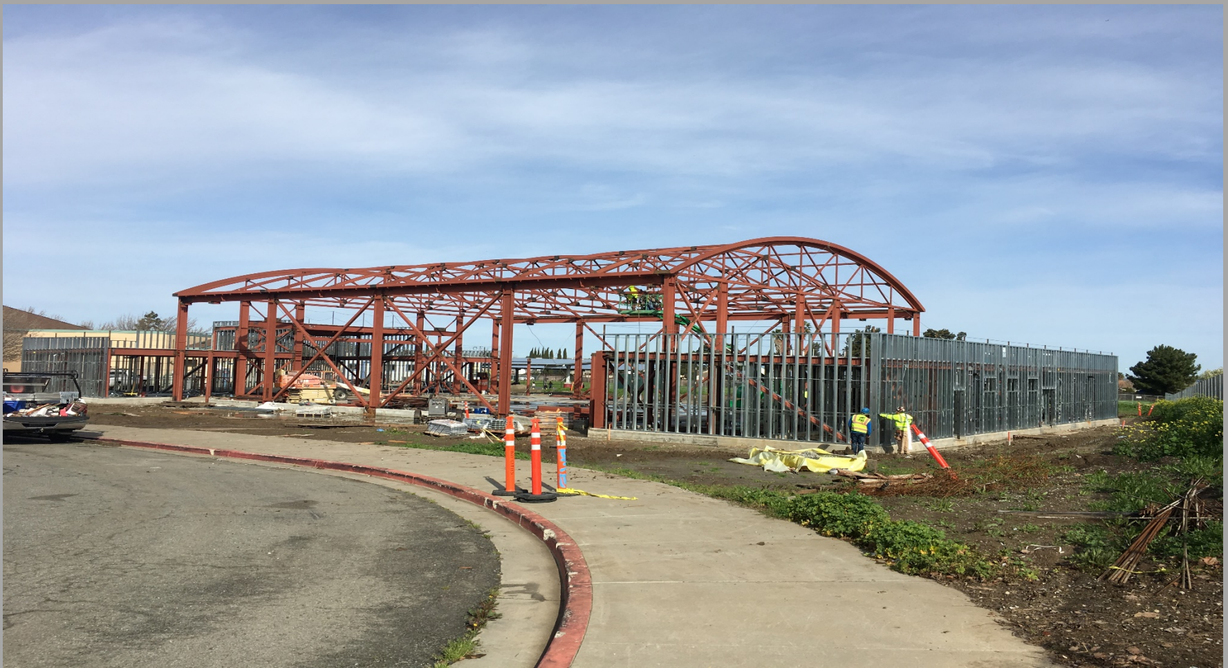
New Gym./MP Bldg. Roof Trusses in place & Exterior Walls Framing Ongoing - Looking Northwest
