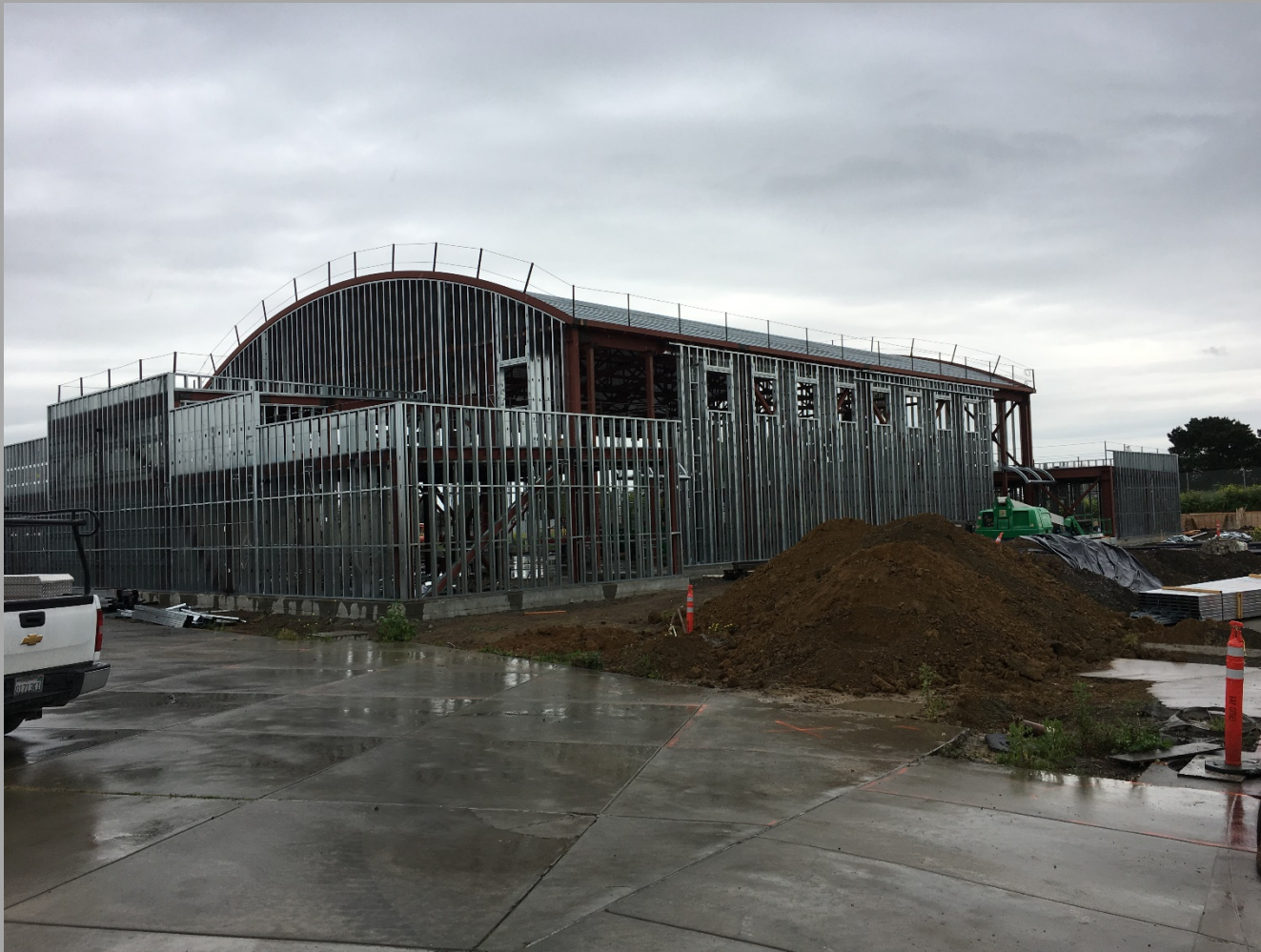
New Gym/MP Bldg. Roof Decking Complete & Exterior Walls Framing Nearly Complete- Looking Northwest
