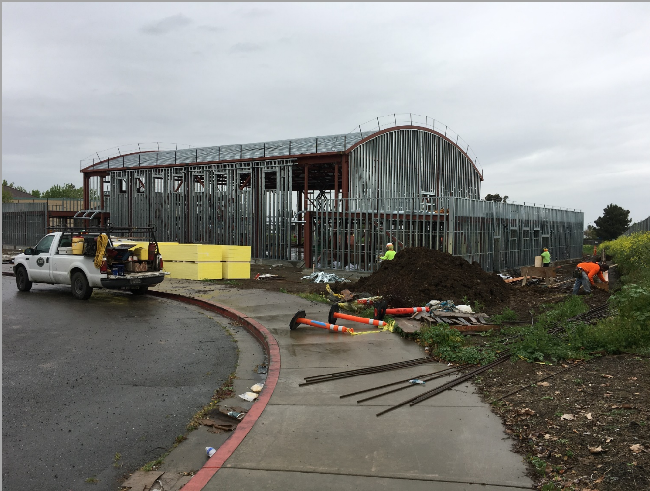
New Gym/MP Bldg. Roof Decking In Place, Exterior Walls Framing Nearly Complete. Retaining Wall Formwork– Looking Northeast
