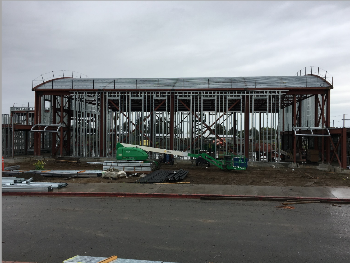
New Gym/MP Bldg. Roof Decking In Place & Exterior Walls Framing Nearly Complete- Looking North
