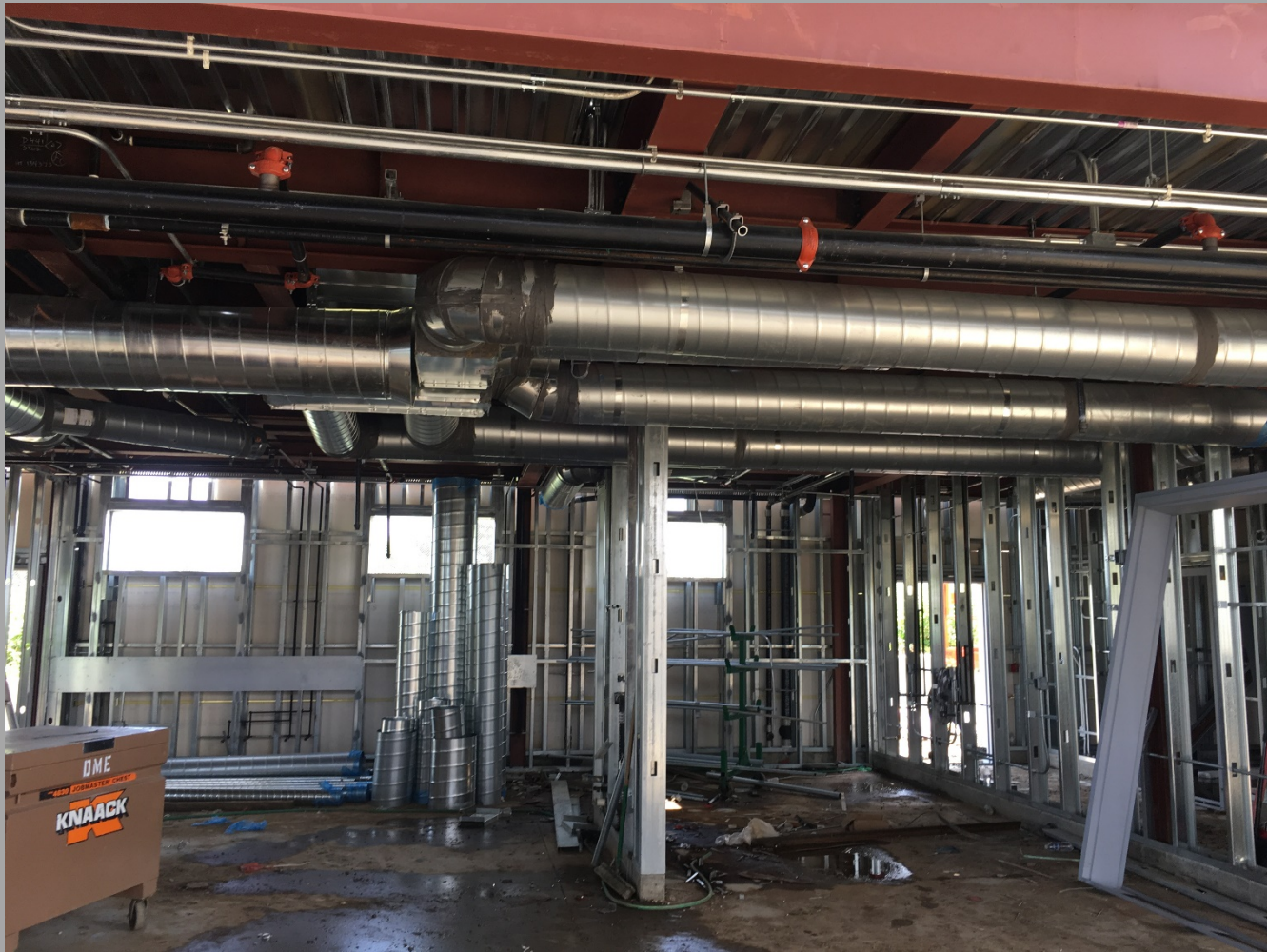
New Gym/MP Bldg. HVAC Duct Work In Place Above Kitchen
