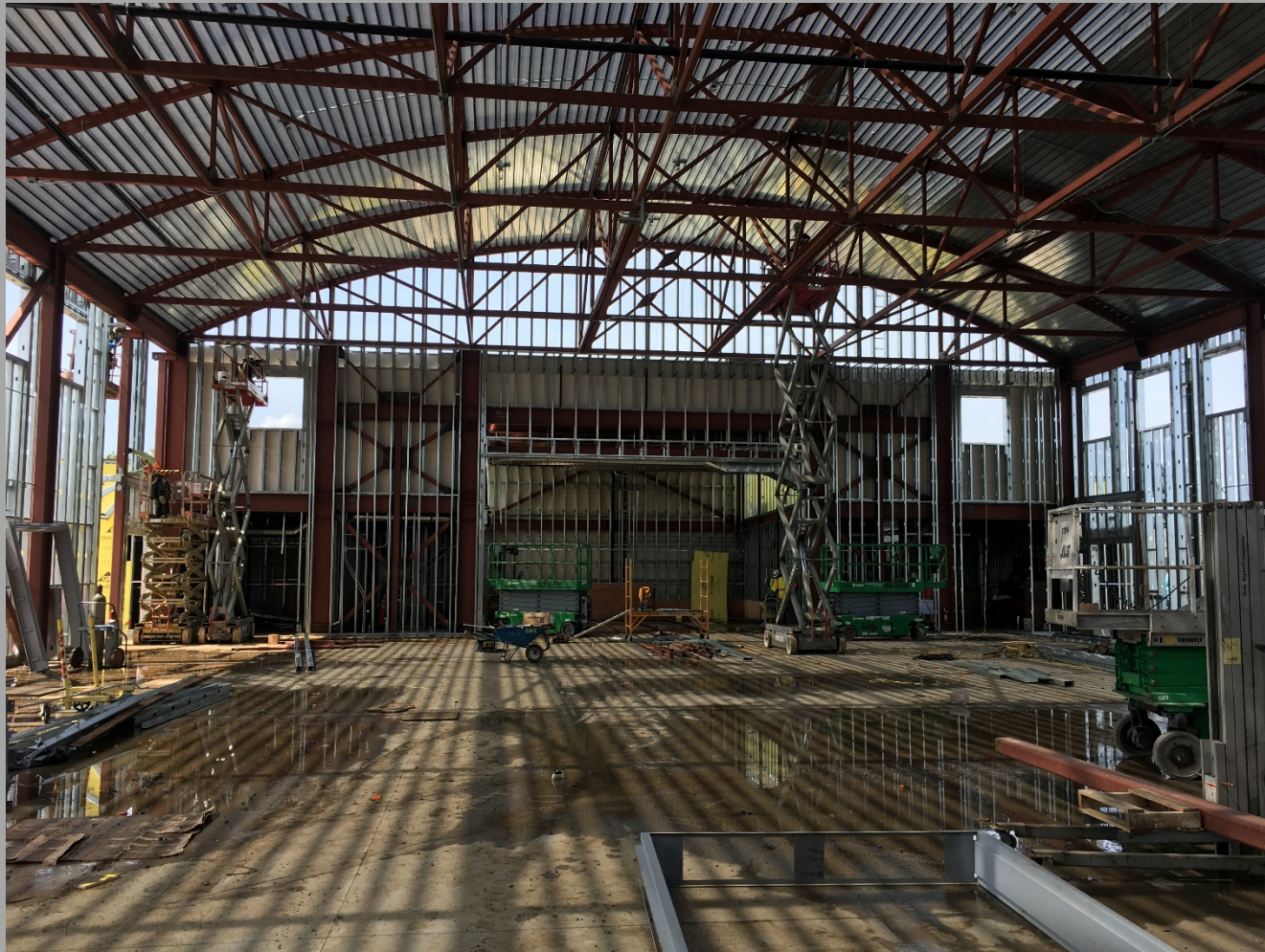
New Gym/MP Bldg. View Of Wall Framing At Platform End Of Building
