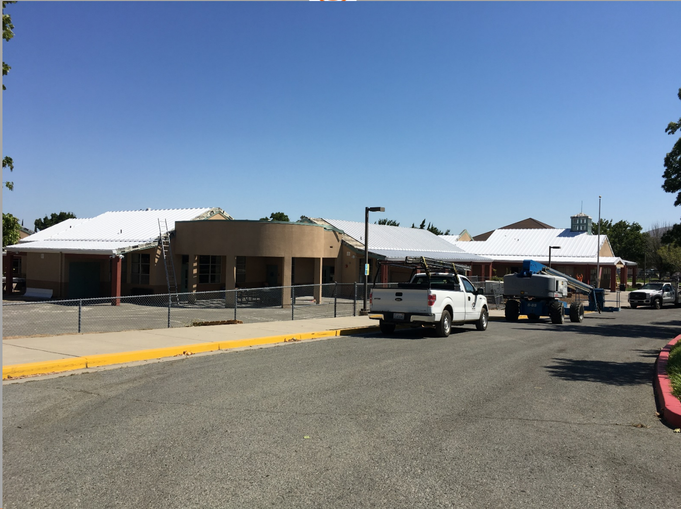
View of New Metal Roofing at Existing School Looking Northeast
