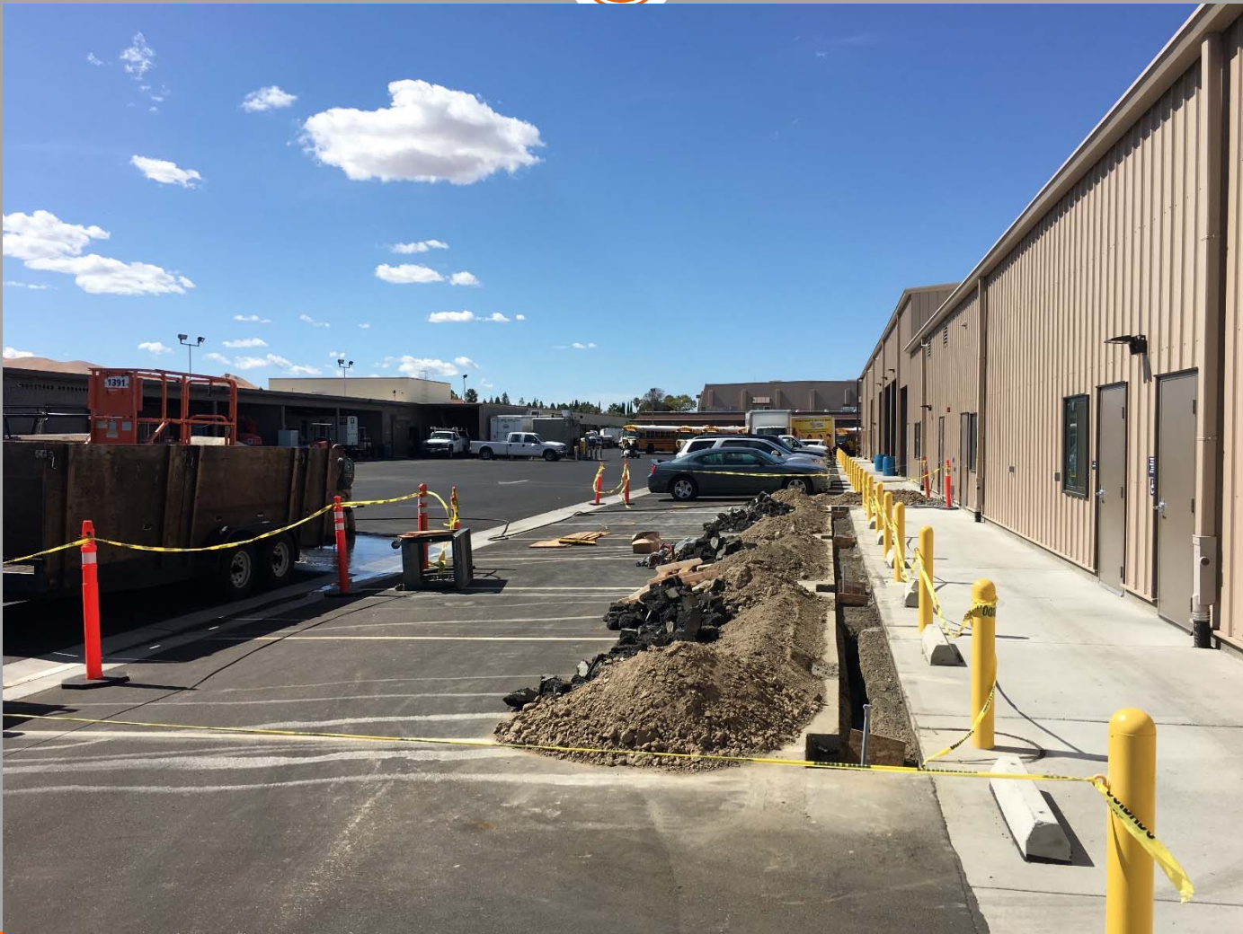
View of Underground Electrical Feed for Charging Stations
