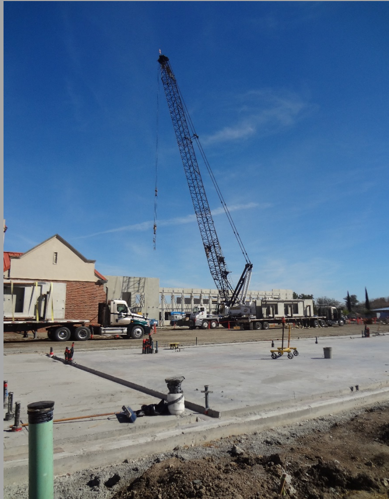
View Of Exterior Wall Panels In Place For New 12 Classrooms Bldg. (Bldg. N1) & West End Of Slab For Building N3
