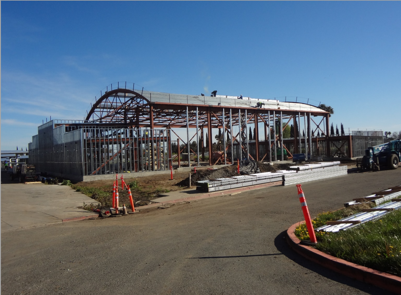
New Gym./MP Bldg. Roof Decking being installed & Exterior Walls Framing Ongoing- Looking Northeast
