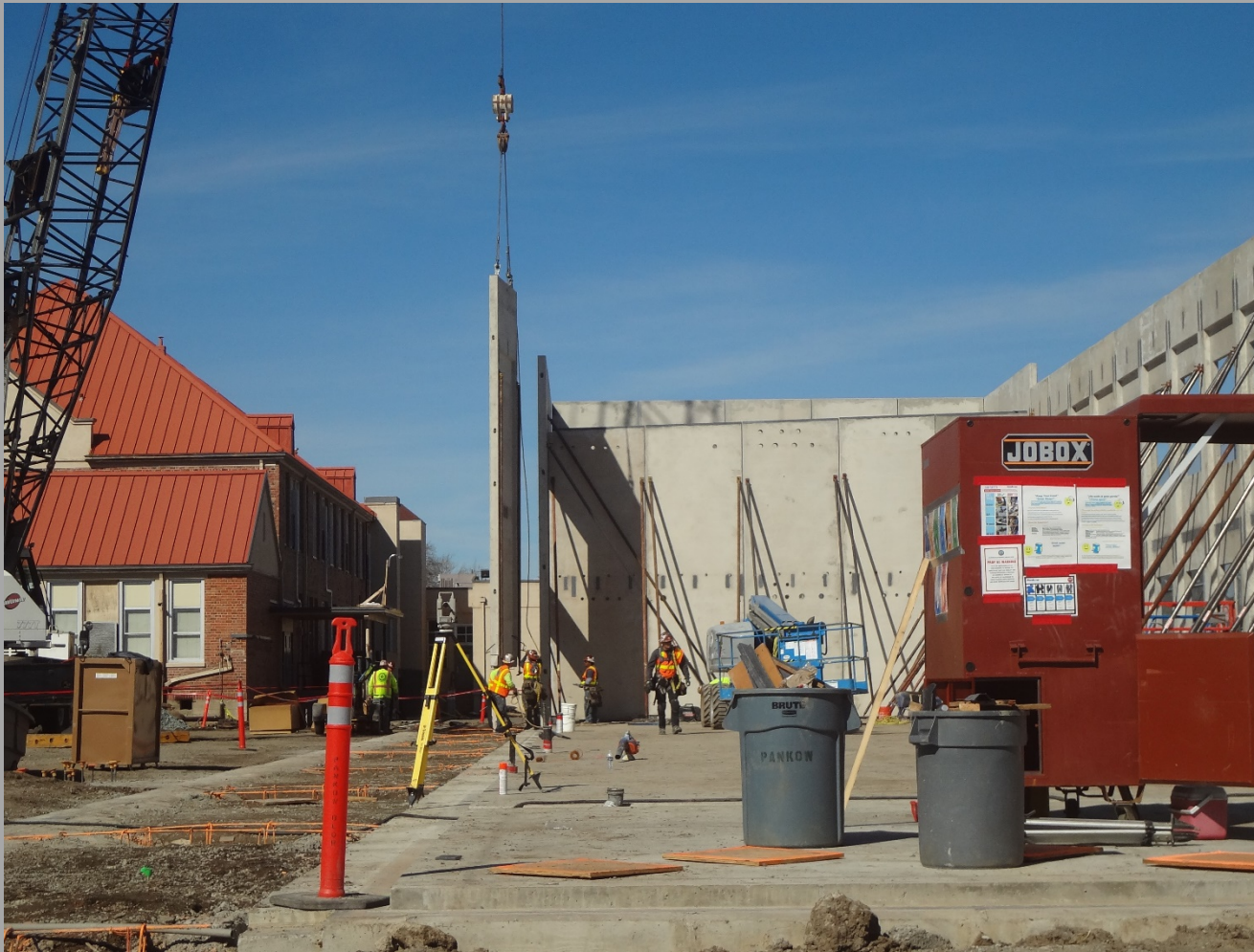
New 12 Classrooms Bldg. (Bldg. N1) South Exterior Wall Panel Being Put Into Place
