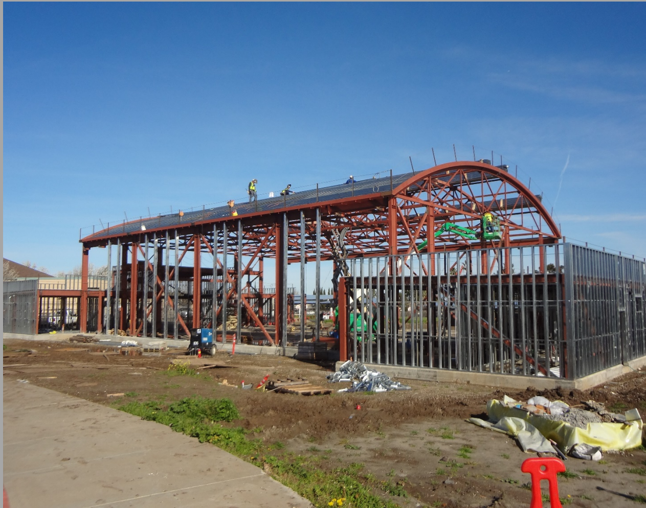
New Gym./MP Bldg. Roof Decking and Exterior Walls Framing Installation Ongoing- Looking Northwest
