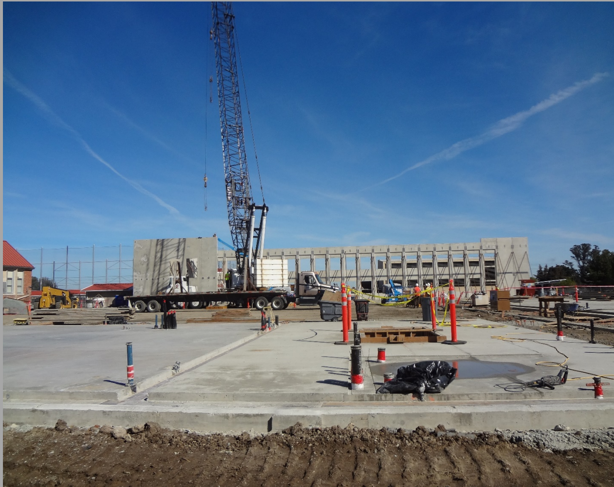
View Of Exterior Wall Panels In Place For New 12 Classrooms Bldg. (Bldg. N1) & East End Of Slab For Building N3
