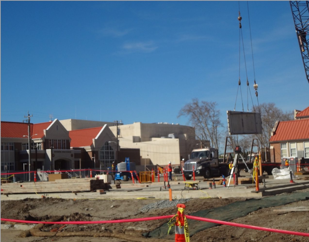
New 12 Classrooms Bldg. (Bldg. N1) Exterior Wall Panel Being Unloaded & Craned Into Place
