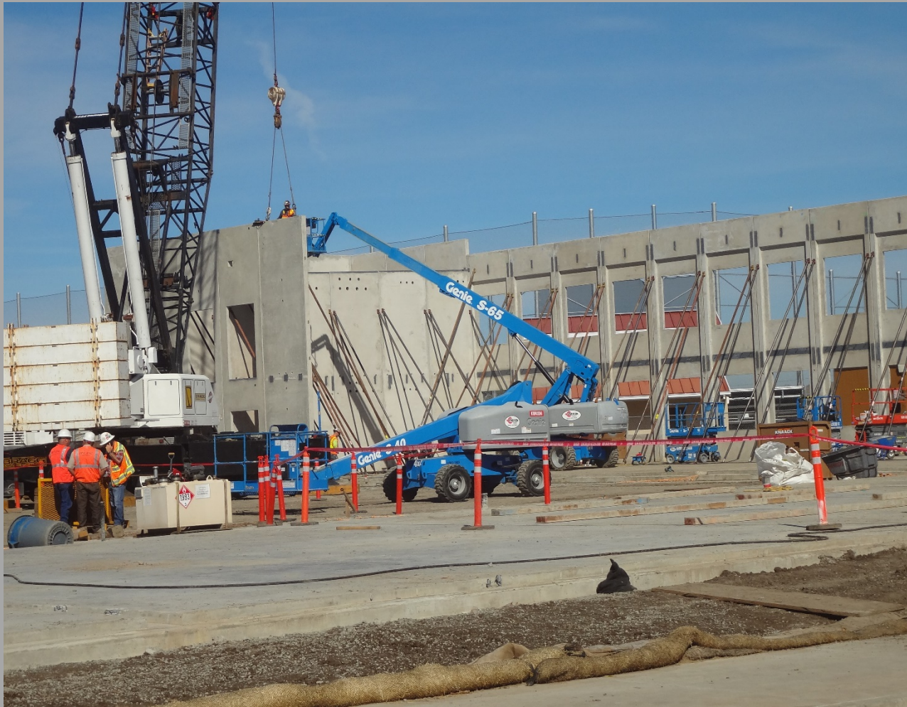
New 12 Classrooms Bldg. (Bldg. N1) South Exterior Wall Panel In Place & Being Levelled
